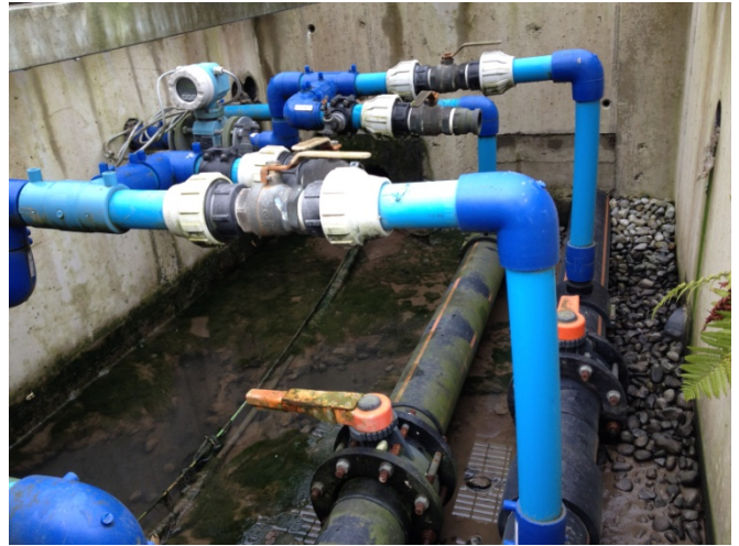
Photograph 12: Pipework for Cells 6 & 8
