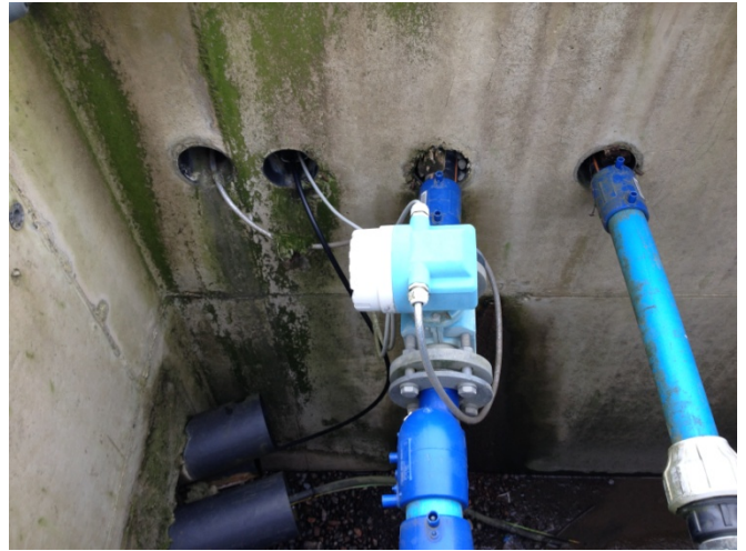
Photograph 9: Pipework at Cells 5 & 7
