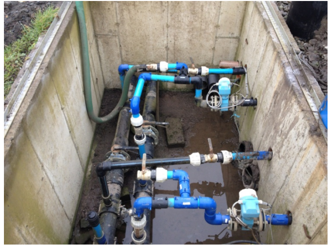
Photograph 16: Pipework at Cell 9 & 11
