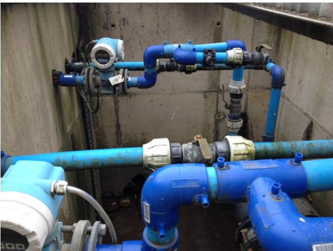
Photograph 10: Pipework at Cells 5 & 7
