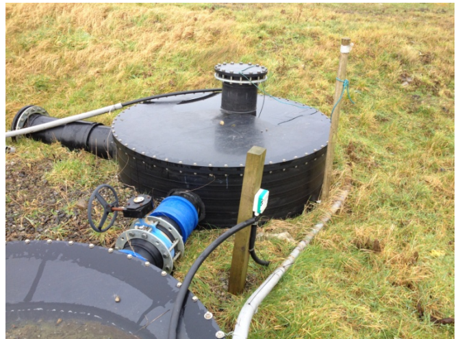
Photograph 21: Insulated condensate pipework
