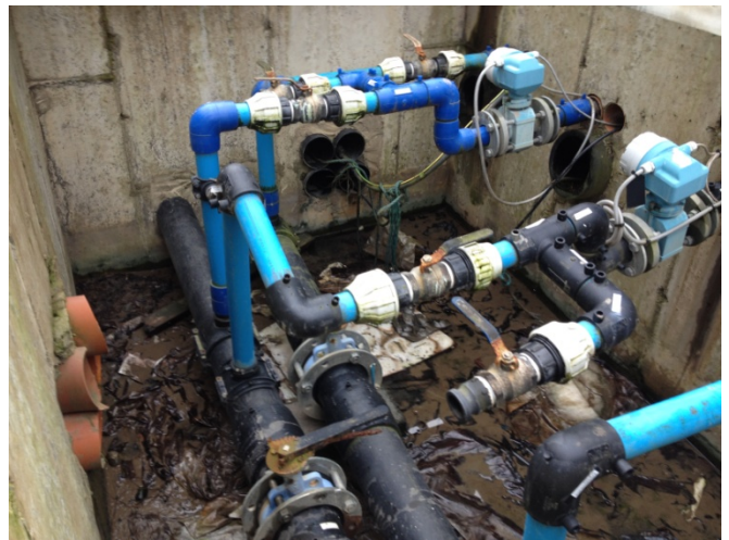
Photograph 18: Pipework at Cell 10
