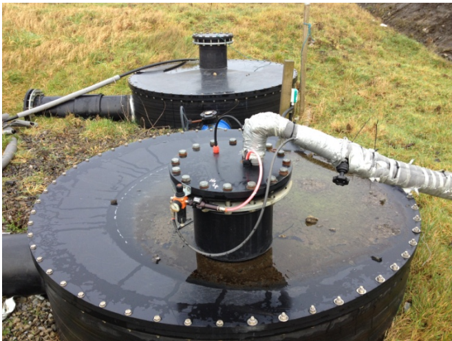
Photograph 20: Insulated condensate pipework
