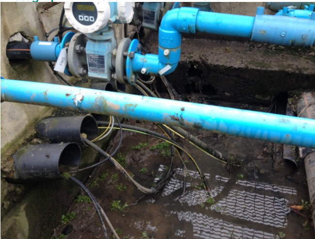
Photograph 3: Pipework in Chamber 1 & 3
