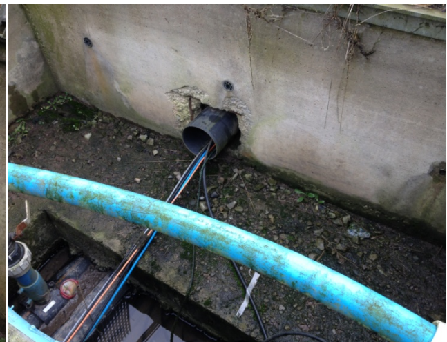
Photograph 7: Pipework for Cells 2 & 4
