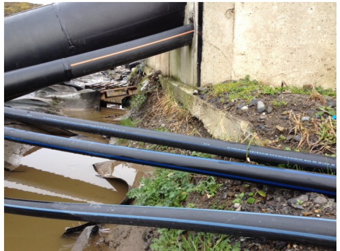
Photograph 14: Undermining to rear of headwall
