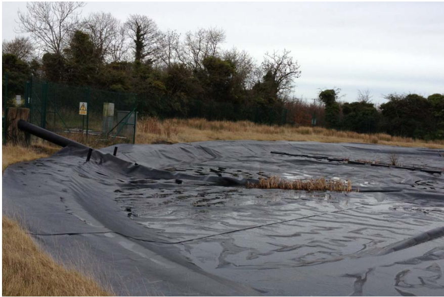
Figure 2.3: Extraction Pipe at lagoon cover
