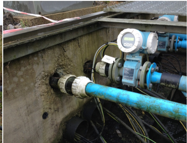
Photograph 5: Concrete damage (construction stage finish)
