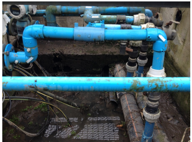
Photograph 2: Pipework in Chamber 1 & 3
