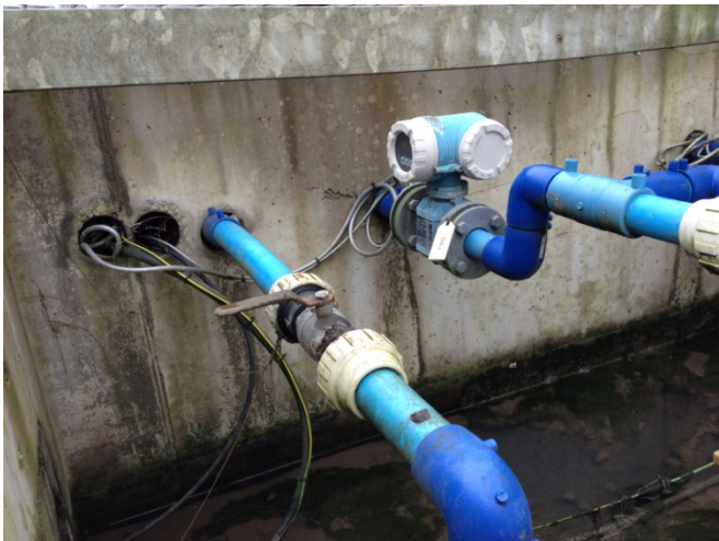
Photograph 13: Pipework for Cell 8
