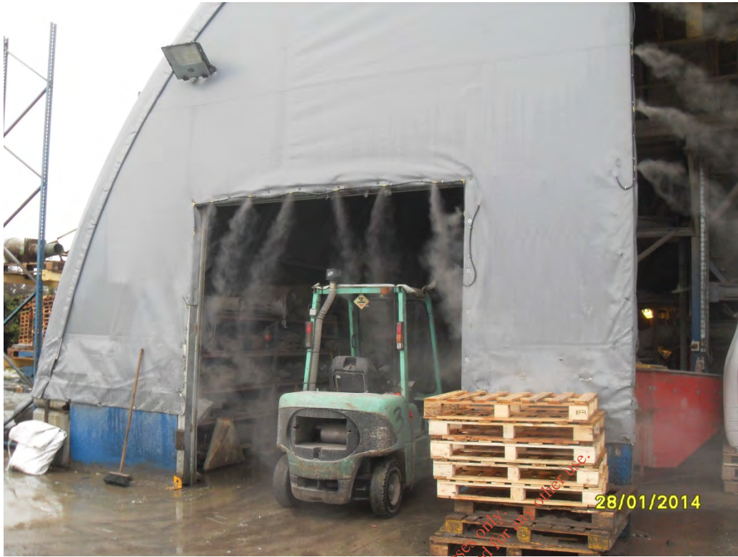
Photograph 5: Misting system at Drying Plant (3)
