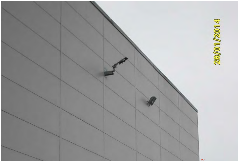
Photograph 1: Water gun #1 positioned at Main Process building
