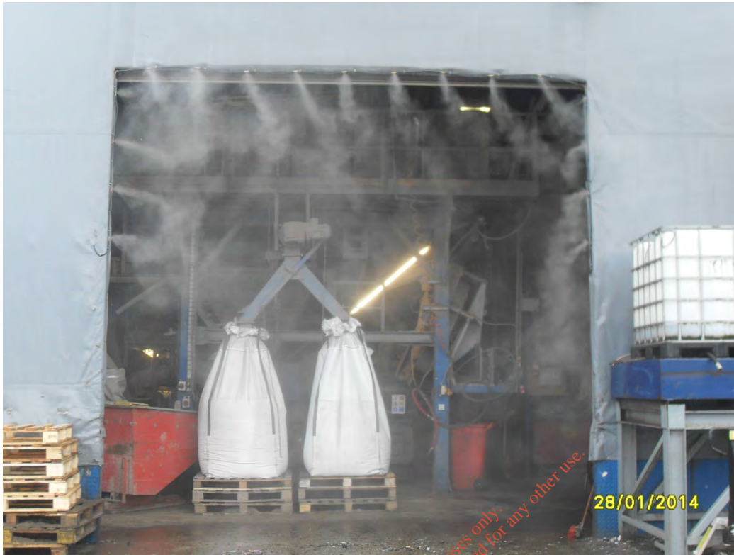
Photograph 3: Misting system at Drying Plant (1)
