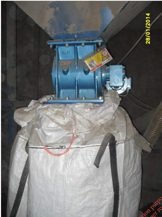
Photograph 9: Sealed/contained chutes/silos to storage bags in Drying Plant (2)
