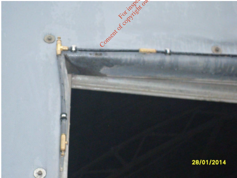
Photograph 6: Misting system at Drying Plant (4) – spray nozzles
