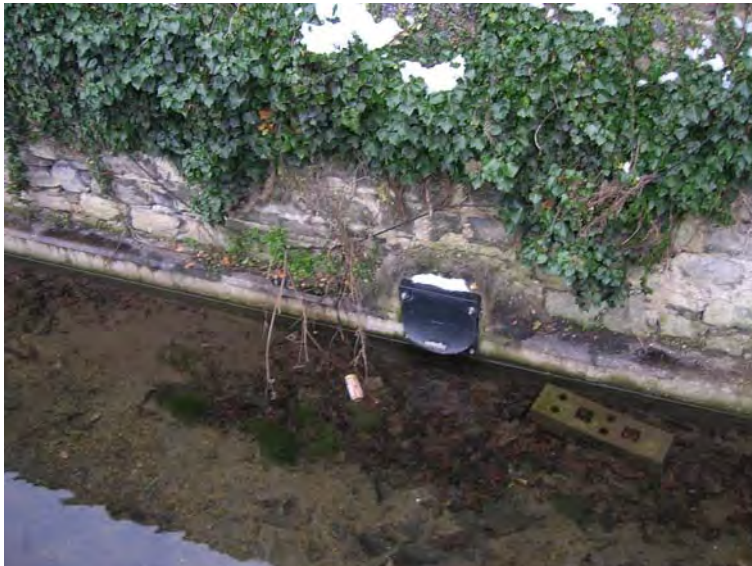
Fig. 18 SWO 13: flap valve at the outfall point.
