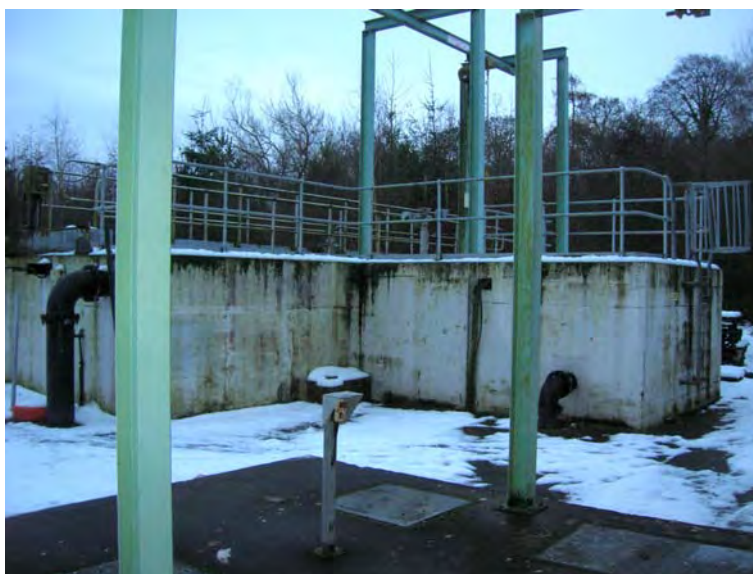
Fig. 2 SWO 2: storm water holding tank
