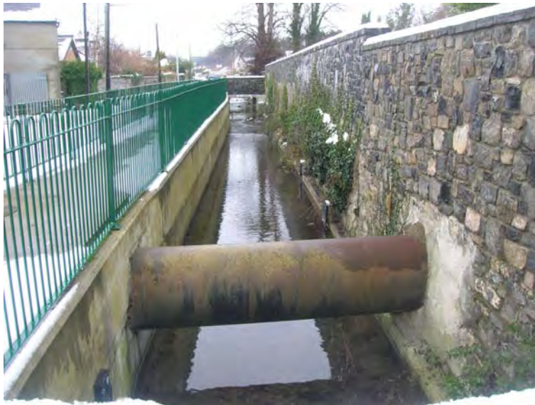
Fig. 19 Silleachain Stream at Mill Lane. SWO 13 visible behind 750mm diameter crossing sewer, at the right.
