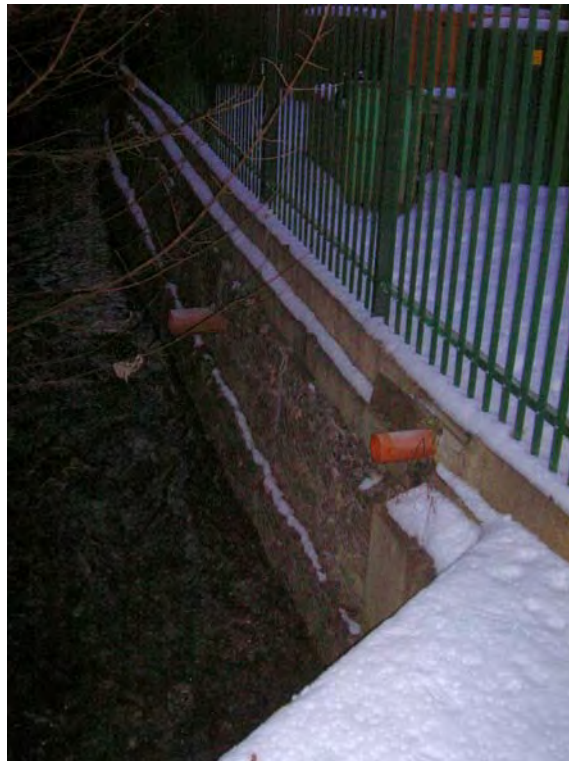
Fig. 15 SWO 11 (150mm pipe, foreground) and SWO 10 (225mm pipe, background)
