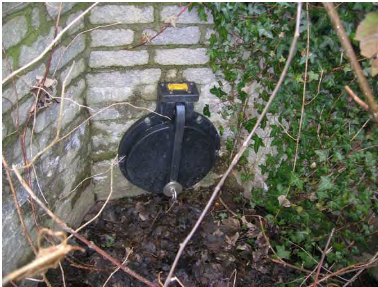
Fig. 20 SWO 14 – flap valve at outfall pipe
