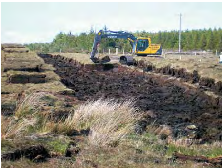
Plate 12.4: Removing turves in intact blanket bog habitat traversed by the Bord Gáis Mayo to Galway Gas Pipeline in the Glenturk More Bog NHA.
