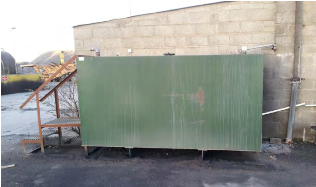
Photo 5 Waste Oil Tank at Back of Maintenance Shed
