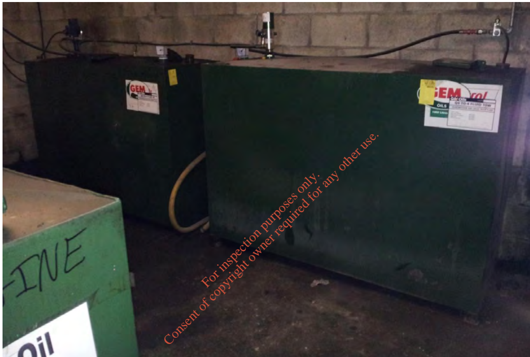
Photo 4 Hydrocarbon Tanks in Maintenance Shed
