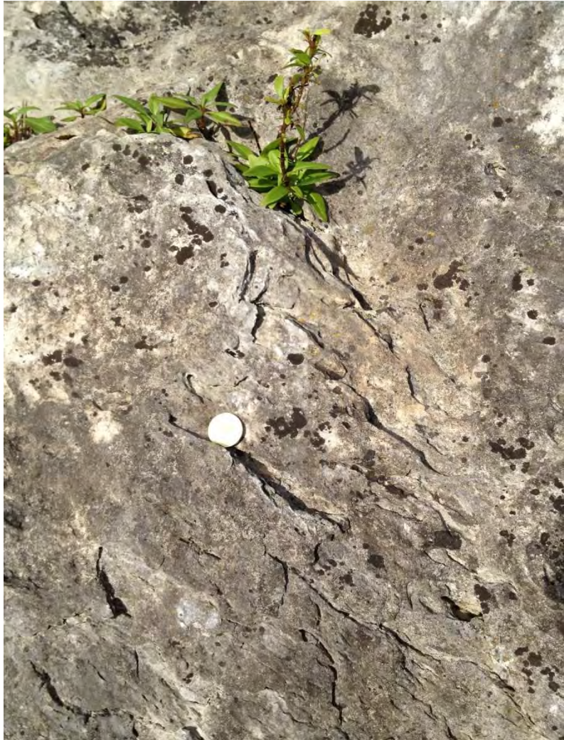
Photograph 13.6: Exposed Limestone Bedrock on “The Island” Bridge Crossing to Haulbowline Illustrating Small Scale Karst Formation on the Surface of the Limestone
