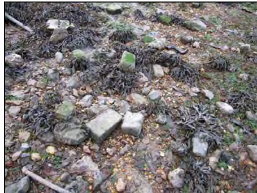
Plate 16: Detail shot of foreshore composition at NGR: 179590E, 65573N, note dislodged stonework from adjacent embankment present at this location.
