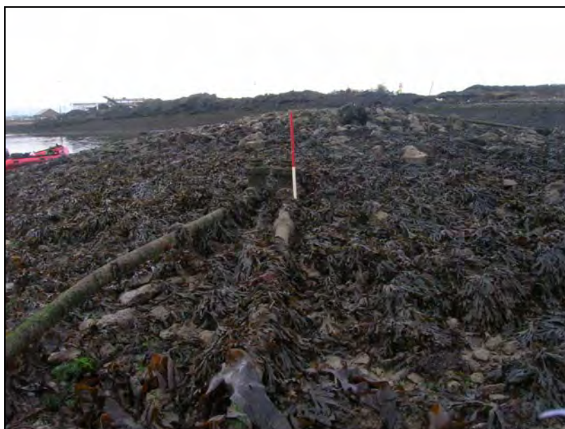
Plate 26: North-facing view of steel-pipe arrangement inserted at the toe of causeway feature (NGR: 179862E, 65180N) and interpreted as a modern service pipe (1m scale).
