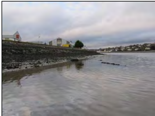
Plate 15: East-facing view of masonry embankment forming north side of Haulbowline Island, taken from NGR: 179562E, 65636N.
