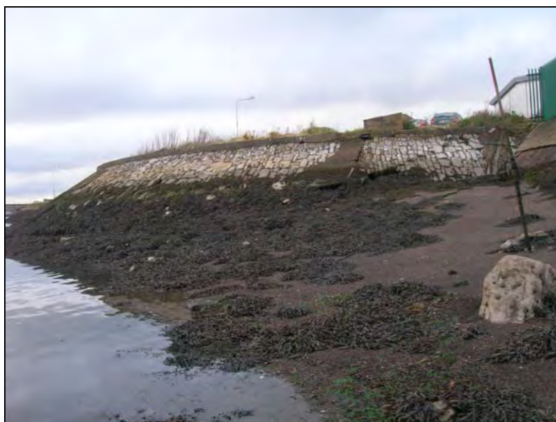
Plate 22: West-facing view of masonry embankment running along south side of Haulbowline Island, adjacent to the dive survey area at NGR: 179482E, 65191N.
