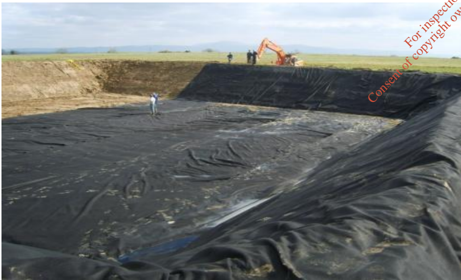
Base cover in position, floats positioned and top shed being rolled out
