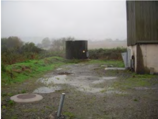
Plate 6: Leachate dilution tank to the north west (behind) the waste transfer station.
