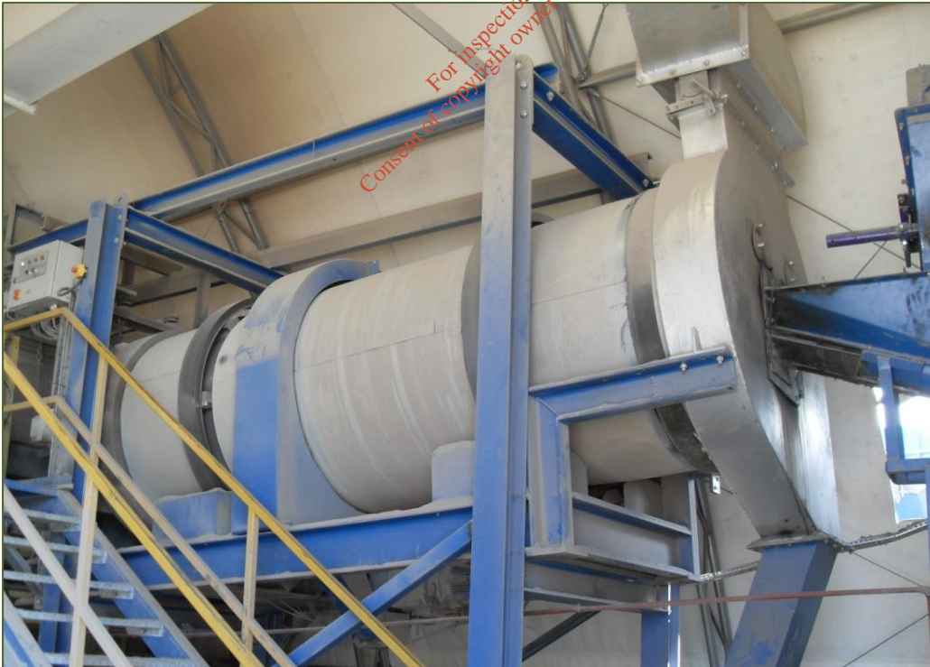
Photograph 2.28: Drying Plant - Rotating Drying Unit
