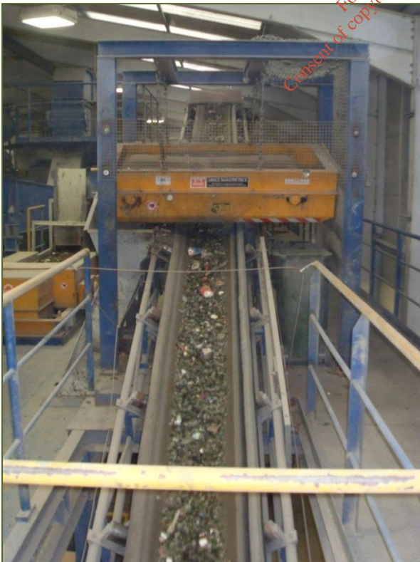
Photograph 2.10: Main Process Building - magnetic separator
