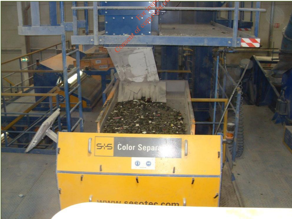
Photograph 2.12: Main Process Building – Spectrum Unit (glass colour separator)
