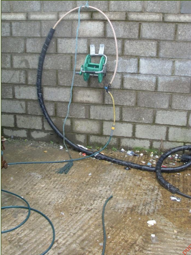
Photograph 2.41: Vehicle wash bay
