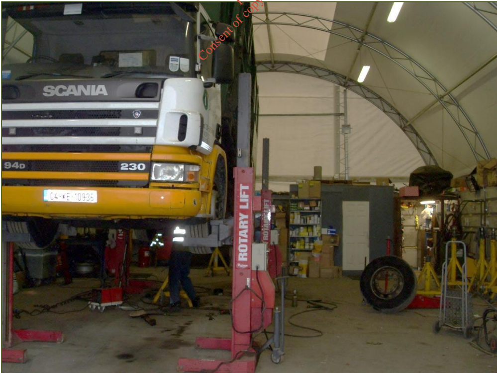
Photograph 2.42: Garage/vehicle workshop plant and equipment
