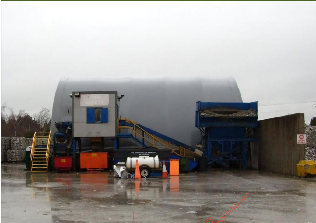
Photograph 2.27: Drying Plant - hopper and picking station
