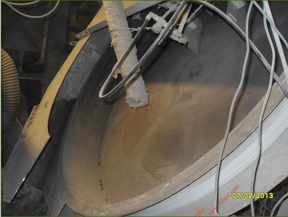
Photograph 2.29: Drying Plant - Pelletiser – Rotating Drum
