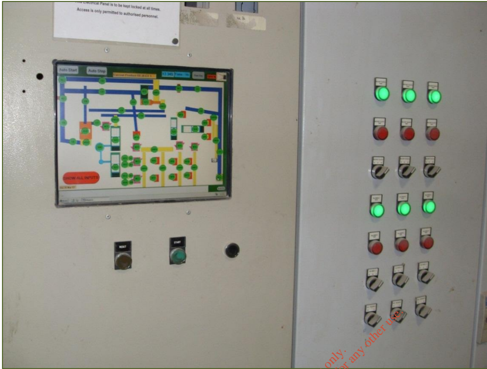
Photograph 2.15: Main Process Building – touch-screen management system
