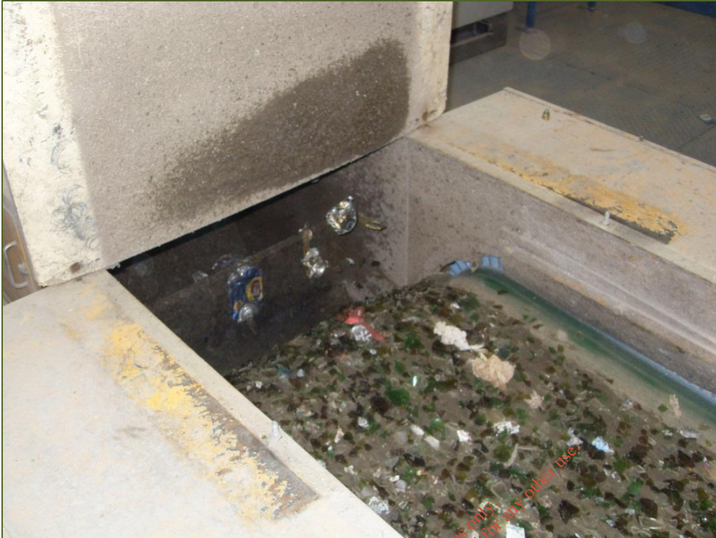
Photograph 2.11: Main Process Building – Eddy Current Separator Unit
