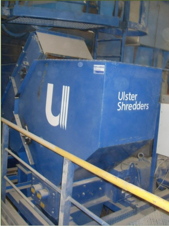
Photograph 2.17: Main Process Building – can shredder
