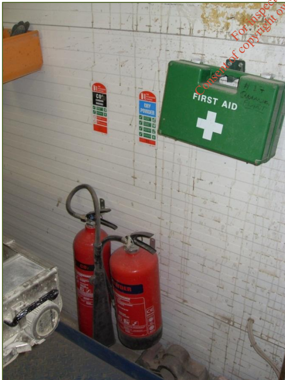
Photograph 2.16: Main Process Building - First Aid/Fire Extinguisher Station
