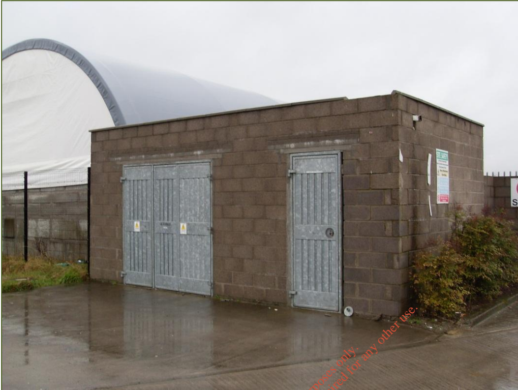
Photograph 2.39: Electricity Sub-station, at Rehab Glassco Site Entrance (outside subject site)
