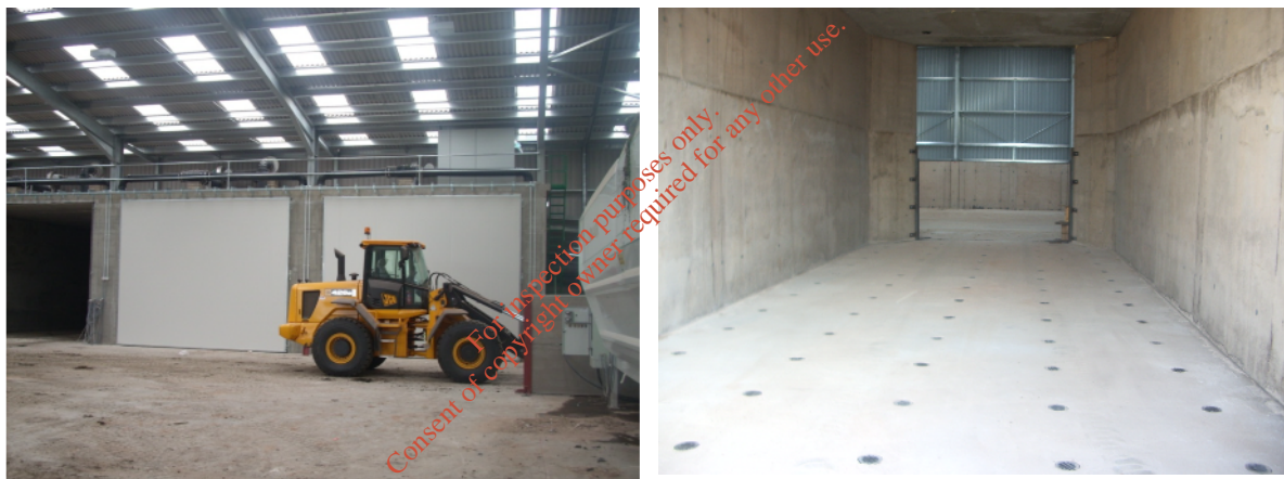
Fig. 14. Exterior of the composting biocells illustrating the sliding doors (left) and the proprietary C:N in-pavement aeration system (right).
