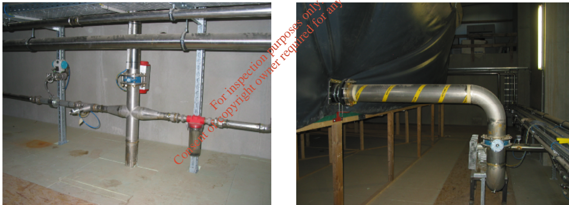
Fig. 12. The pneumatic gas collection system on the roof of the fermenters (left) and the gas transfer blower to the gas bag located in the roof space above the fermenters (right).
