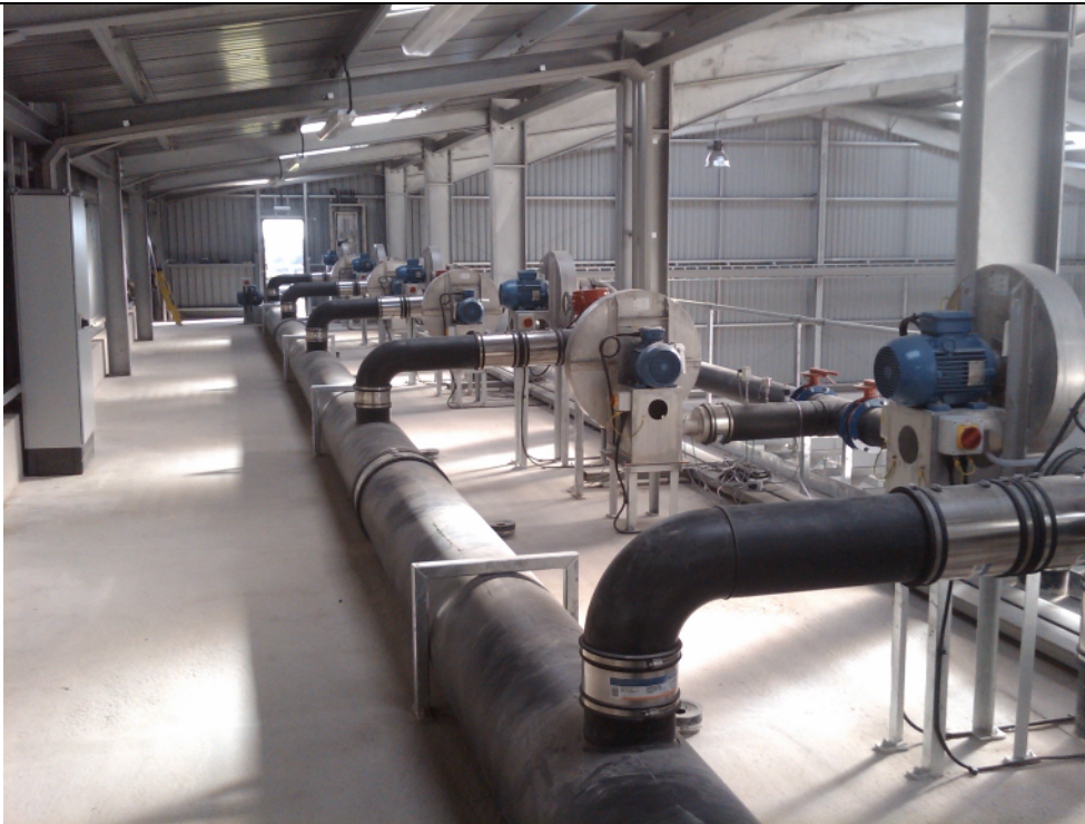
Fig. 17. The blower modules in the gallery of the Deepmoor tunnel composting facility in Devon.
