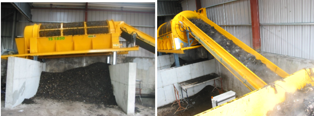
Fig. 18. Housed trommel screen illustrating multiple sections that produce different grades of compost and overs.
