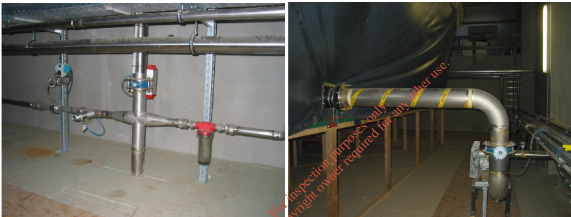
Fig. 13. The pneumatic gas collection system on the roof of the fermenters (left) and the gas transfer blower to the gas bag located in the roof space above the fermenters (right).
