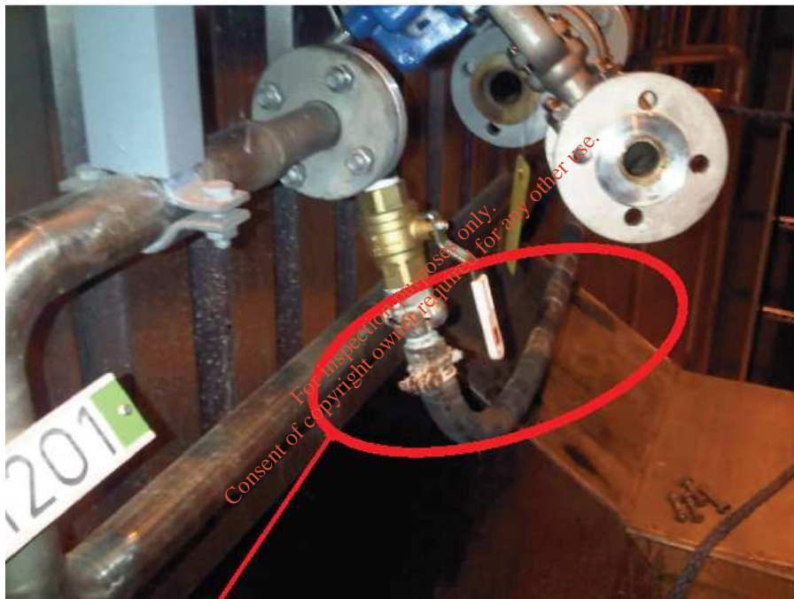
Flexible line from tanker connected into fixed feeding system.
