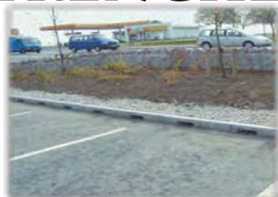
Side-entry pits drain to infiltration trench in car-park
