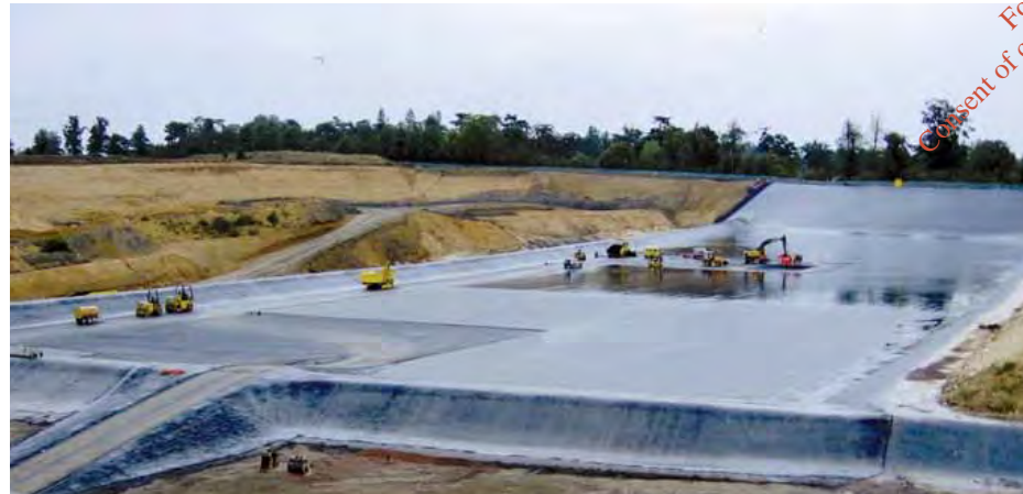
A landfill cell being lined with our impermeable DAC system, even the ramps into the cell can be completely sealed with our DAC and then trafficked.
