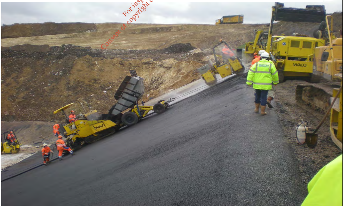
Photo 4 Lining of a side slope with DAC at a UK Landfill Site – note the steepness of the slope
