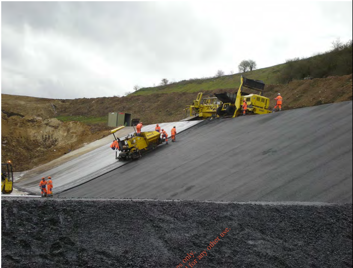
Photo 3 Lining of a side slope with DAC at a UK Landfill Site
