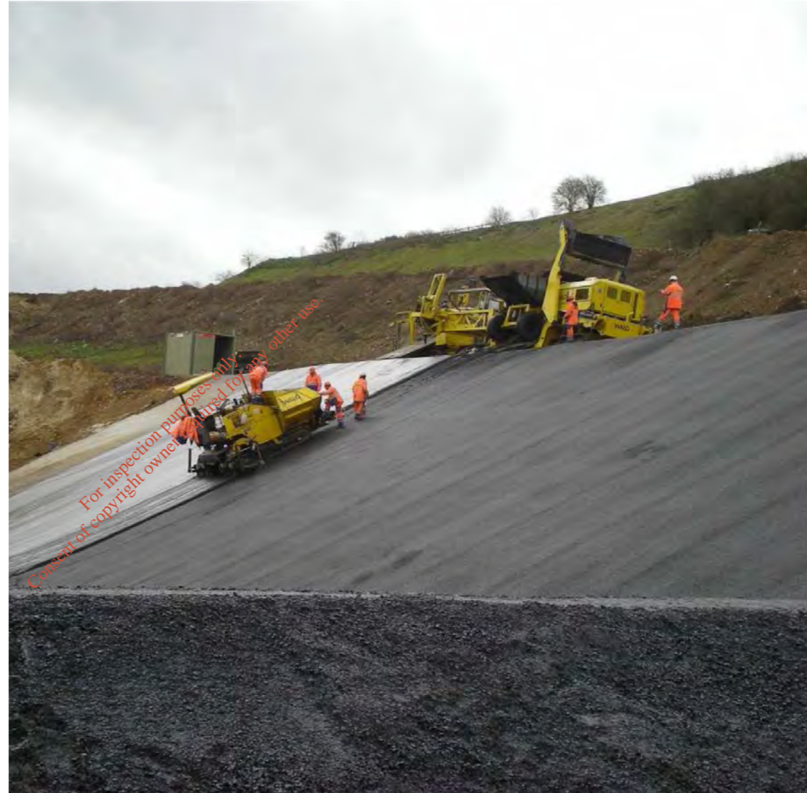
Construction of Dense Asphaltic Concrete (DAC) Liner on side Wall of Waste Cell
