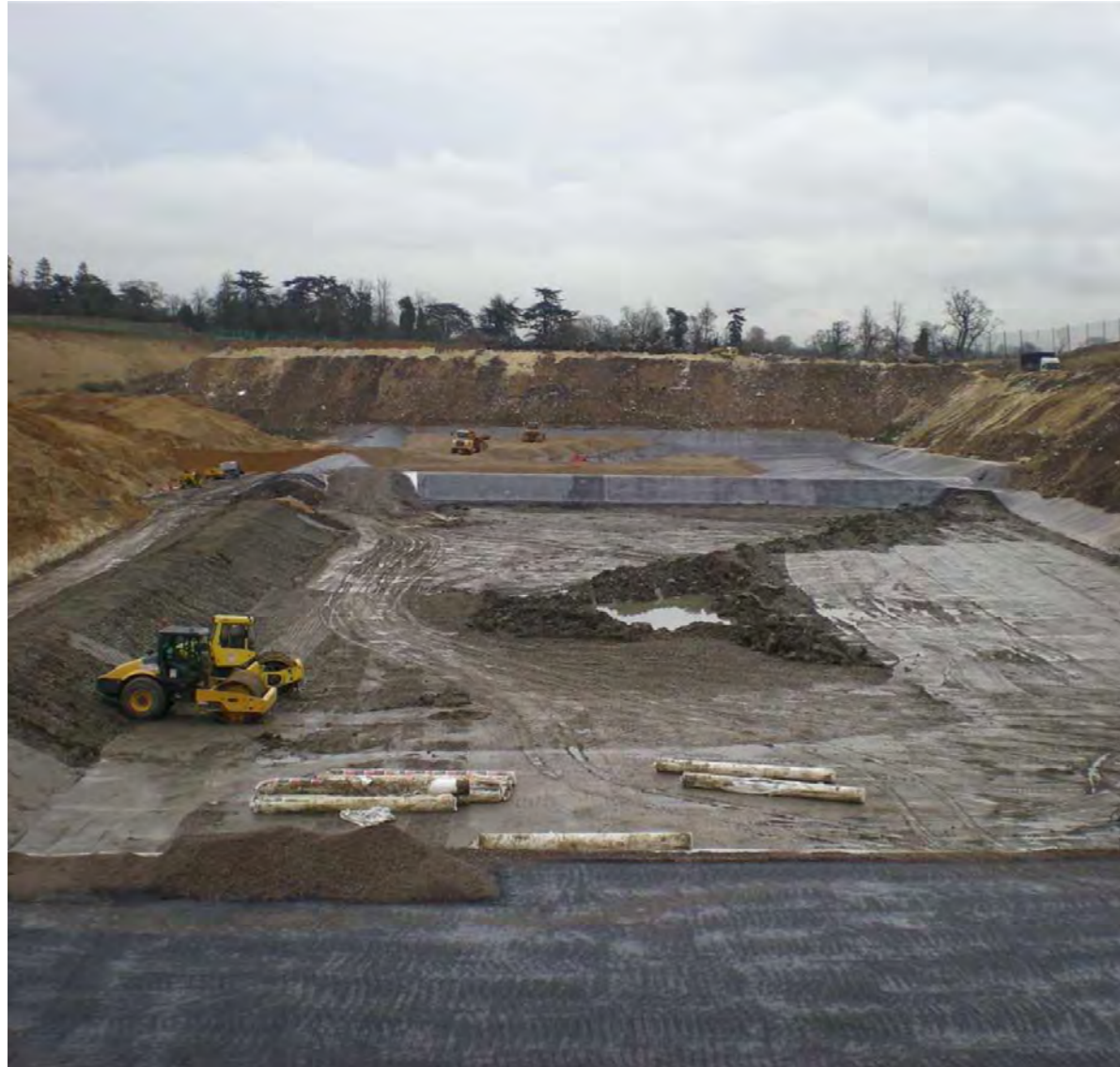
Construction of Dense Asphaltic Concrete (DAC) Liner on base of Waste Cell
