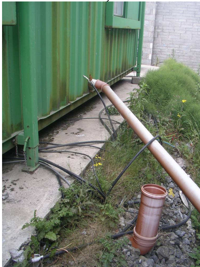
Figure 15: Pipe in ground with high gas concentrations located to the rear of a portacabin in Erin Recyclers.
