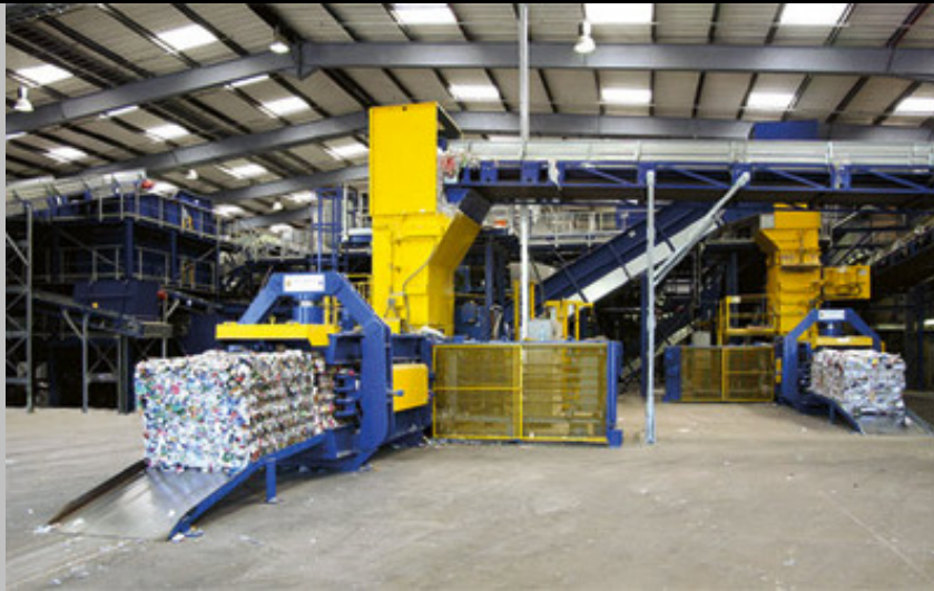
Typical Baler Installation
