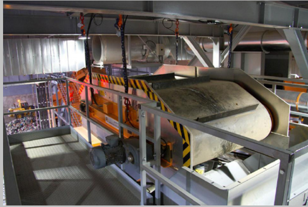
Typical Overband Magnet Installation
