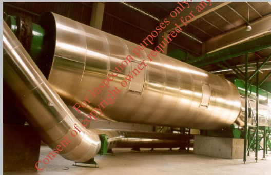
Typical Thermal Drier Installation
