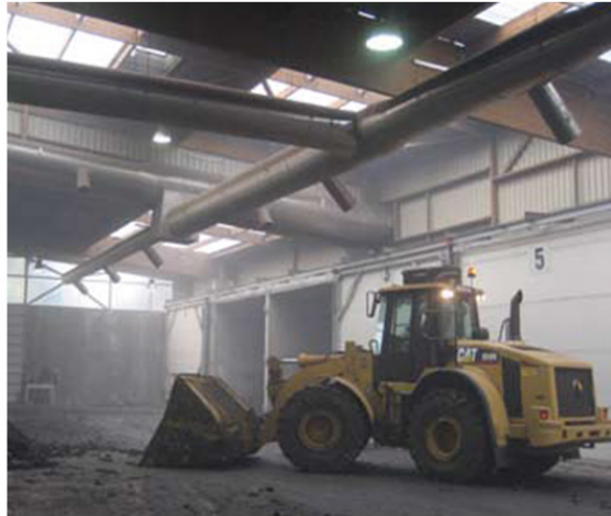
Loading of Dry AD Tunnels
