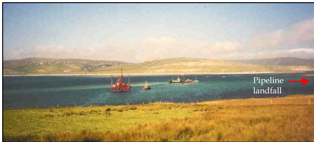
Plate 1. Excavation operations under way in Broadhaven Bay during the summer 2002. The angle of view is approximately northwards from the Glengad site.
