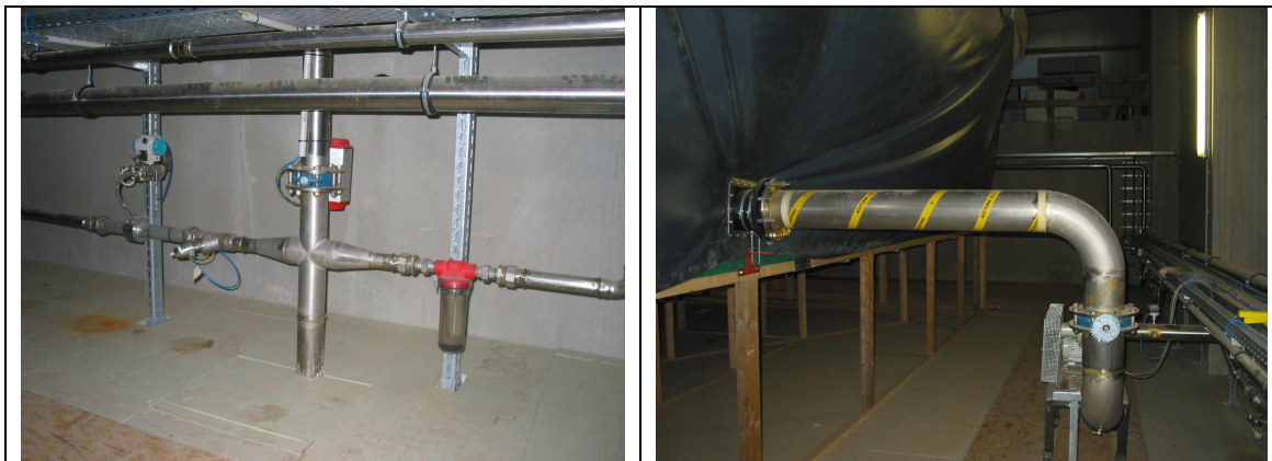
Figure 7 The pneumatic gas collection system on the roof of the fermenters (left) and the gas transfer blower to the gas bag (right).
