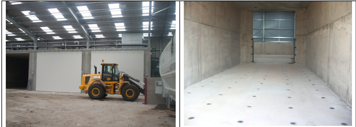
Figure 9 Exterior of the composting biocells illustrating the sliding doors (left) and the proprietary C:N in-pavement aeration system (right).
