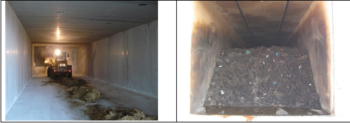
Figure 6 Interior of fermenter prior to filling (left) and with bio-waste prior to fermenter sealing.
