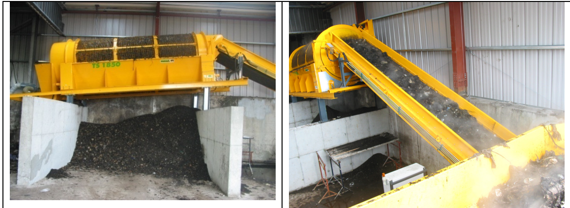
Figure 12 Housed trommel screen illustrating multiple sections that produce different grades of compost and overs.
