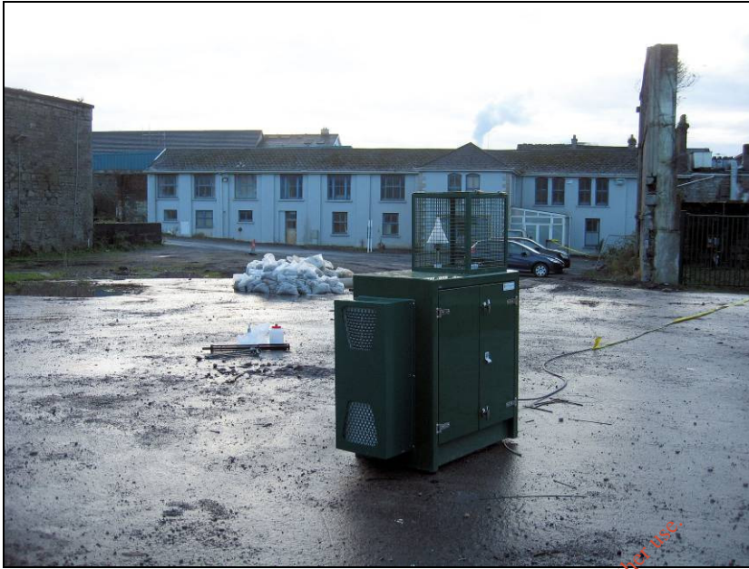
Plate 16: Continuous Monitoring Unit, View 1
