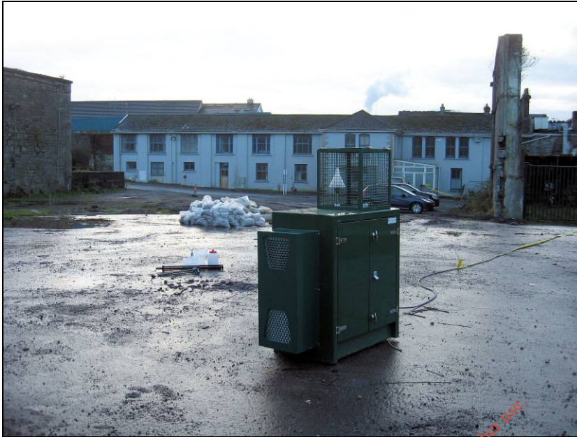
Plate 16: Continuous Monitoring Unit, View 1
