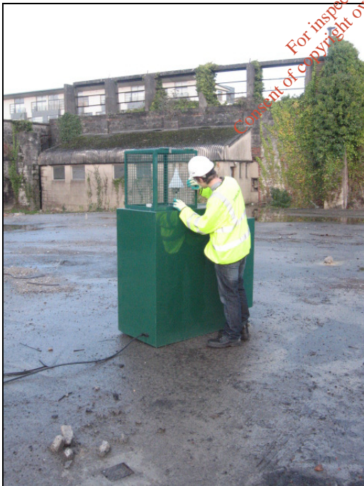
Plate 17: Continuous Monitoring Unit, View 2
