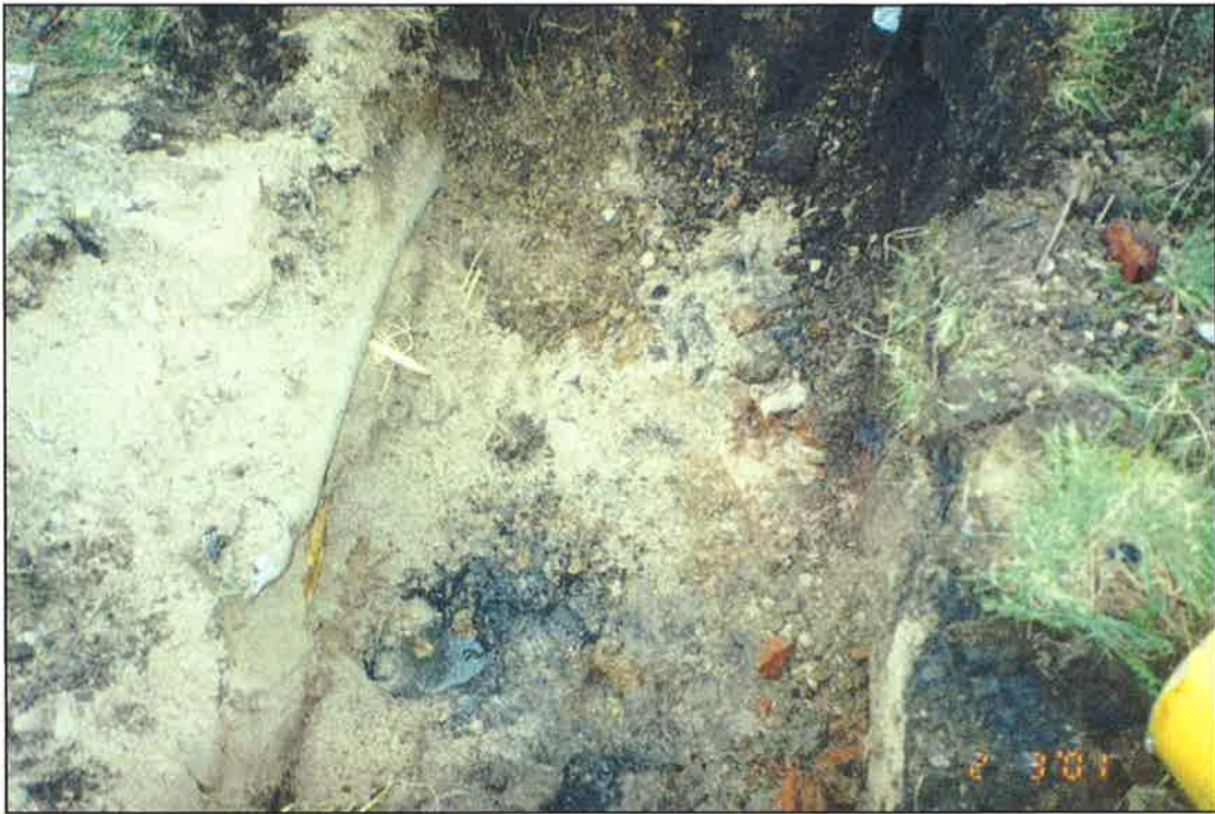
TP 41 View South East Showing Service Duct and Gas Main in Left Hand Side
