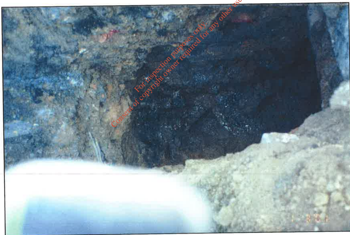
TP 48 View North into Contents of Tank
