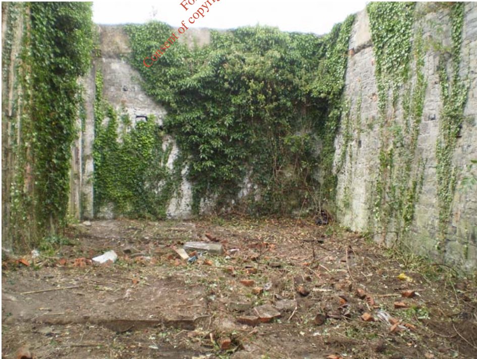
Photo 14) Inside booster house
