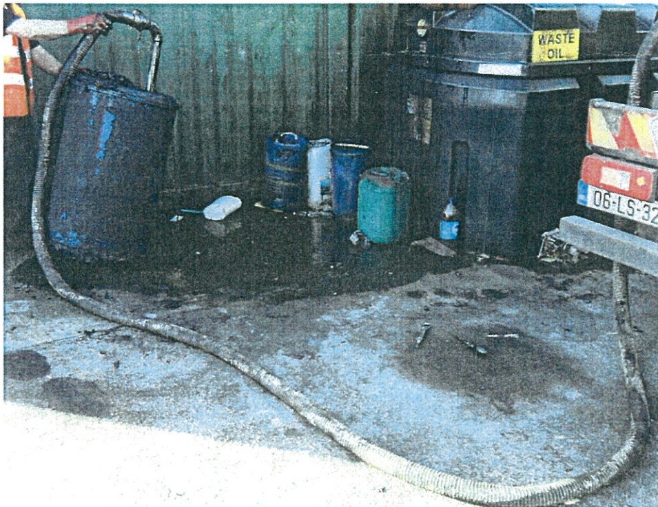
Photo 2: Spillages of oil noted at the waste oil storage area of the civic waste facility.
