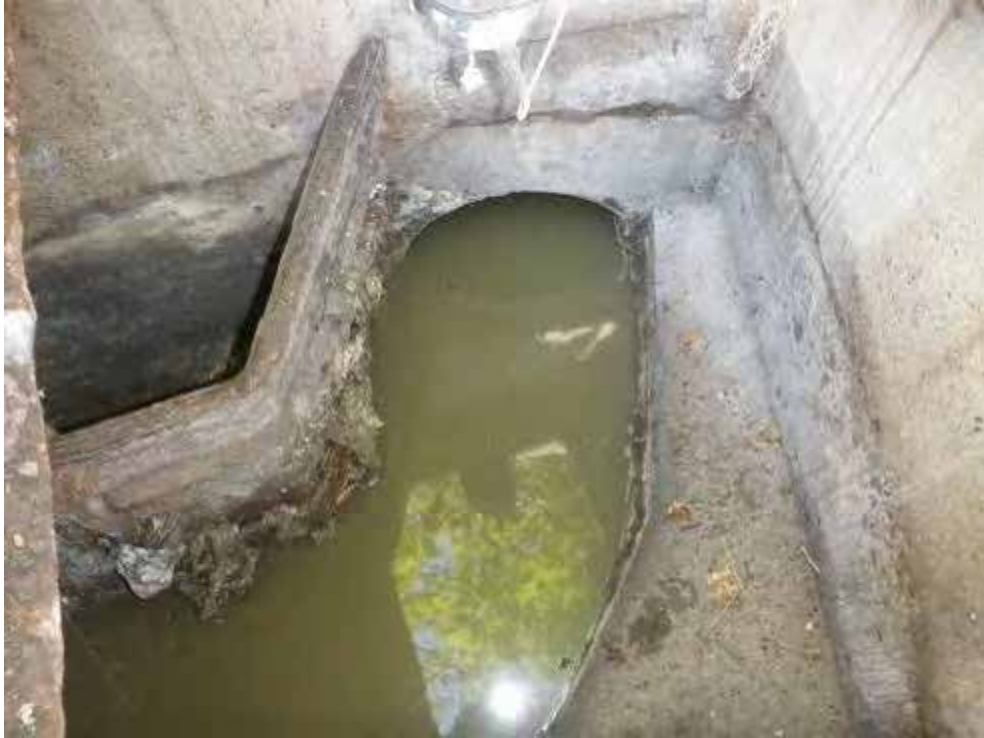
Main Incoming Pipe
