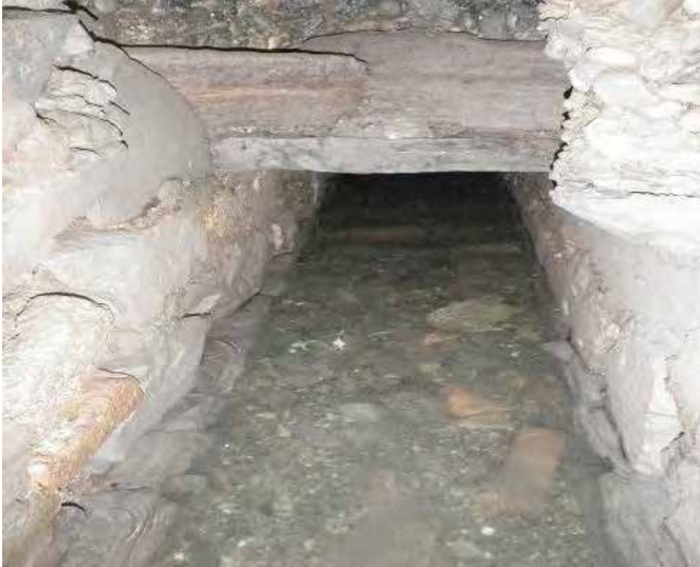
Incoming Surface Water Pipe
