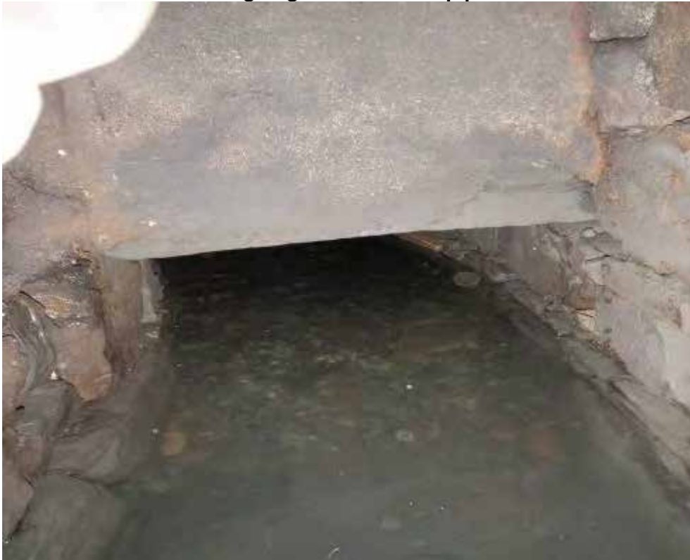
Outgoing Surface water pipe
