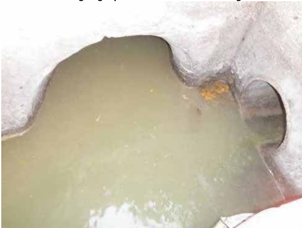
Outgoing Pipe with side 225mm incoming
