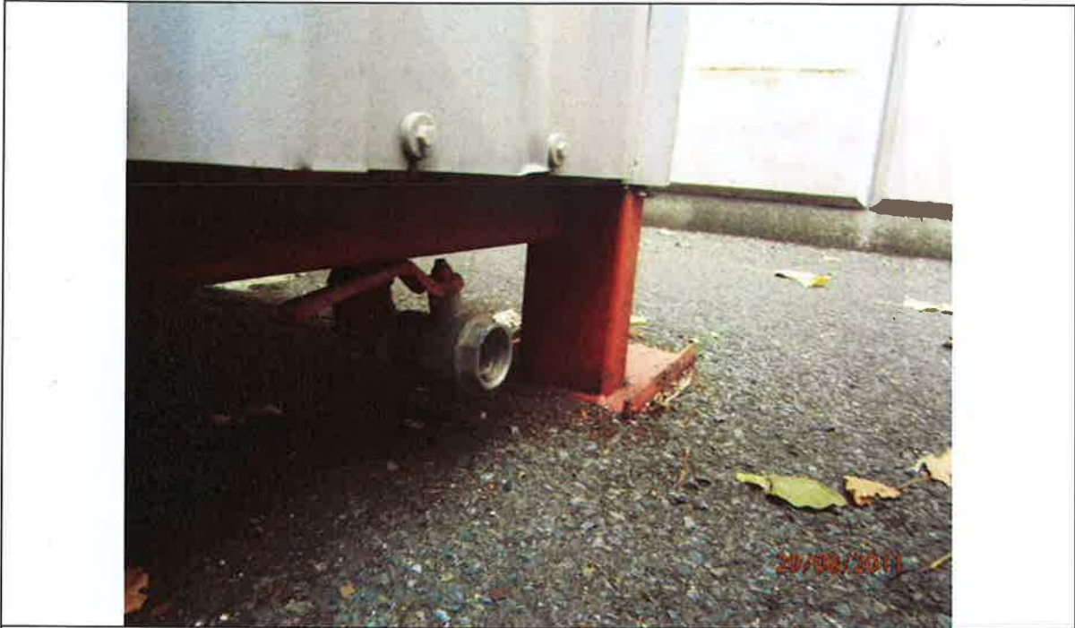
Figure 5.3: Bund 05 – Bund outlet, now with valve
