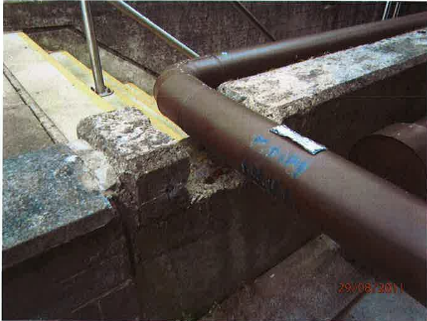
Figure 2.4: Bund 02 – Outlet pipe from CBST 4 running over stairs of ductway
