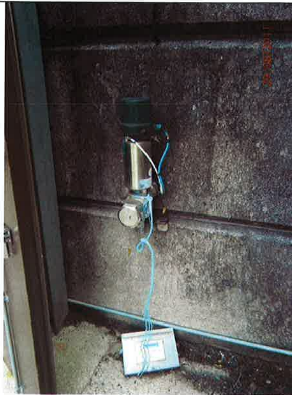
Fig. 23.2: Bund 23 – connection point for delivery, not within containment area
