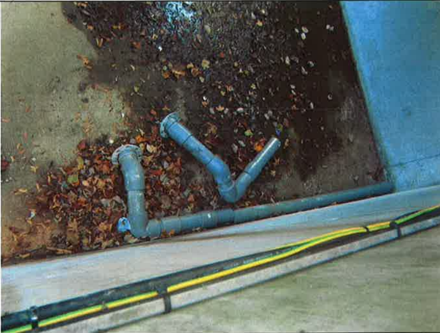
Fig. 37.2: Piping off-cuts in base of bund
