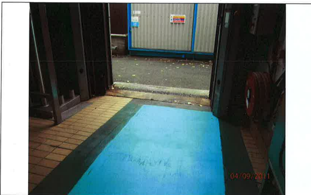
Fig. 32.1: Bund 32 - Slope from Process area to roller door out to yard on south side of site
