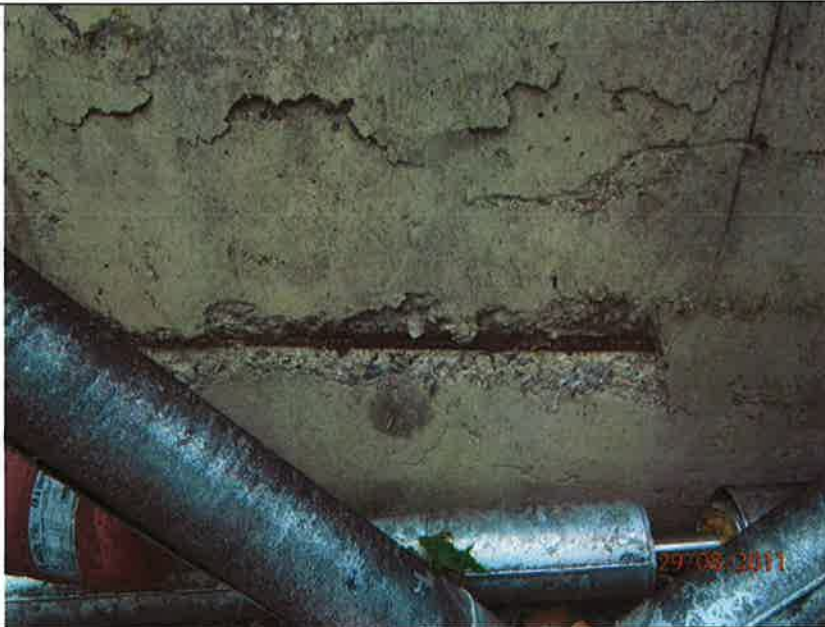
Fig 28.6: Bund 28 – Minor damage to exterior of bund wall on east side
