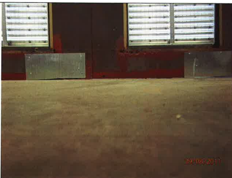
Fig 30.1: Bund 30 - Gaps under door of Sprinkler Pump House
