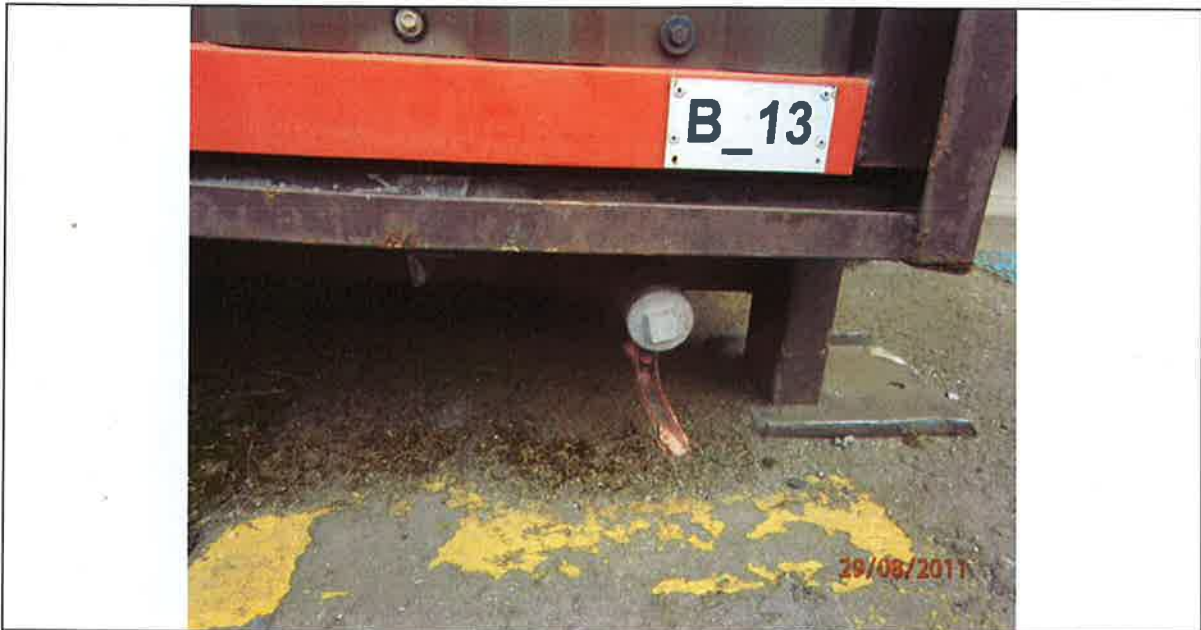
Figure 13.2: Bund 13 – Bottom Outlet Valve: stoppered + with valve
