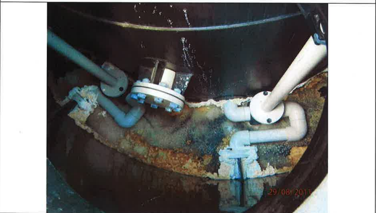
Fig. 7.2: Bund 07 – Liquid caustic retention
