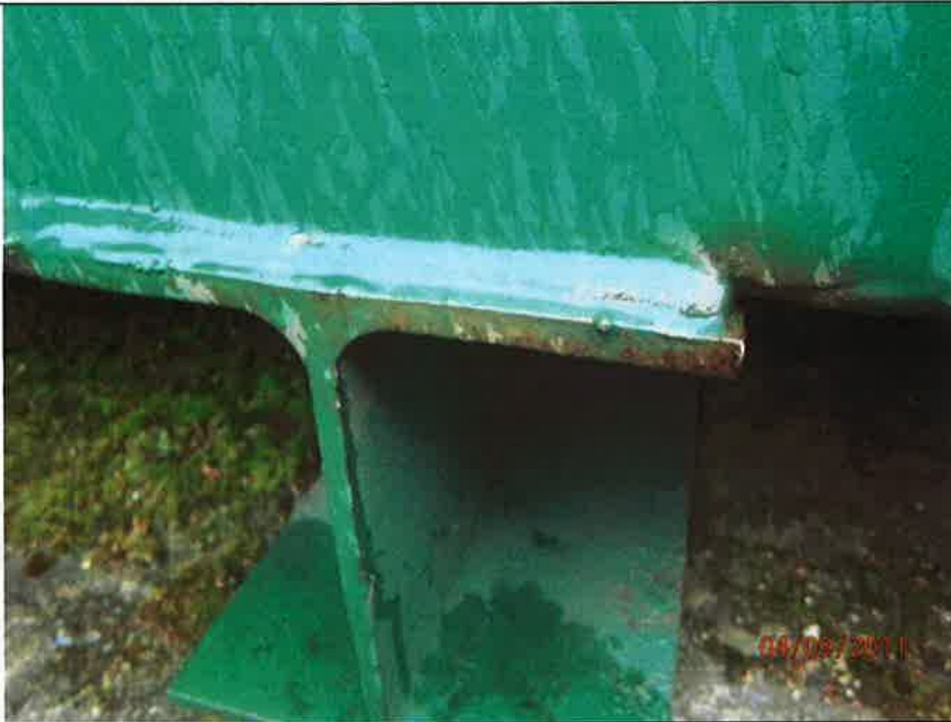
Fig 31.2: Bund 31 - Minor rusting where support welded to tank
