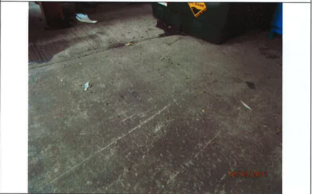
Fig. 38.3: Markings on ground from forklift activity in vicinity of bund
