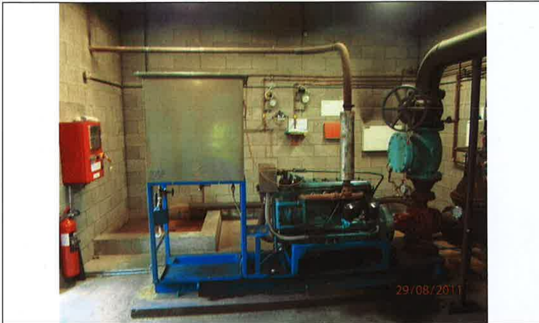
Fig 30.2: Bund 30 – Diesel tank and pump in Sprinkler Pump House
