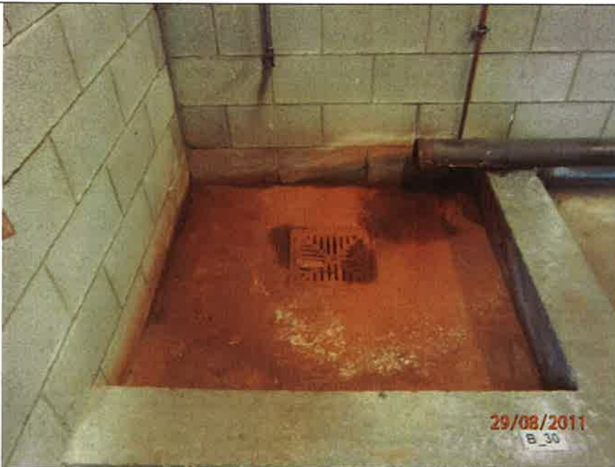
Fig 30.5: Bund 30 – Drain to effluent for water used in sprinkler pump test
