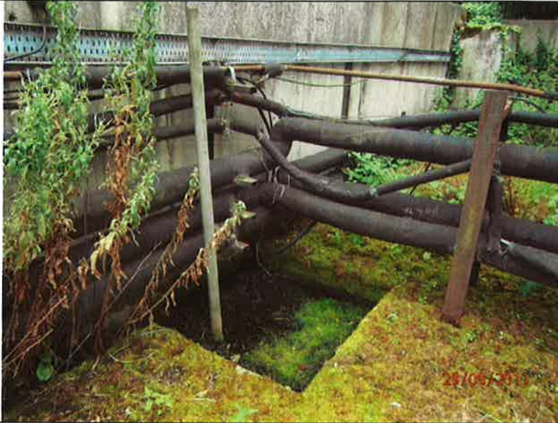
Fig 28.4: Bund 28 – Cabling off cable tray and within sump in bund. Poor condition of pipework also.
