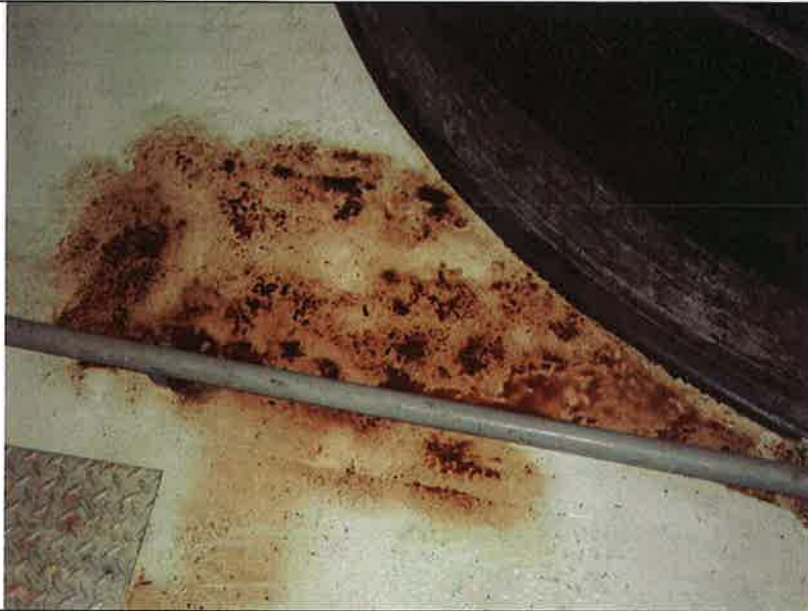
Fig. 26.3: Evidence of leak around the bund
