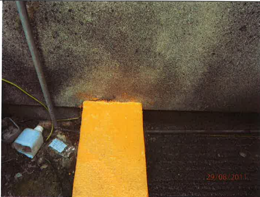
Fig. 20.3: Bund 20 – Cable breach of bund wall
