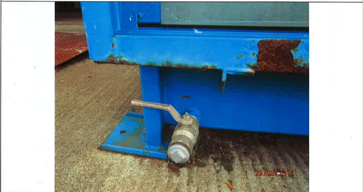
Figure 11.2: Bund 11 – Bottom Outlet Valve of Bund 11
