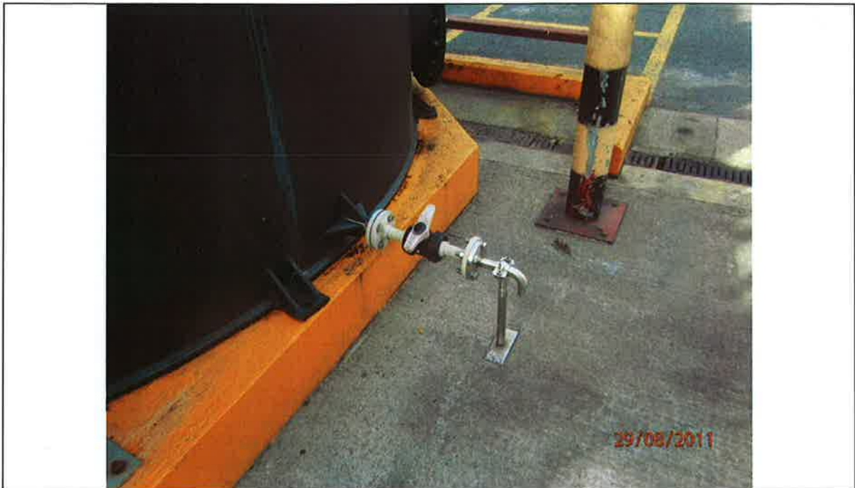
Fig. 9.2: Bund 09 – Bottom Outlet Valve of bund
