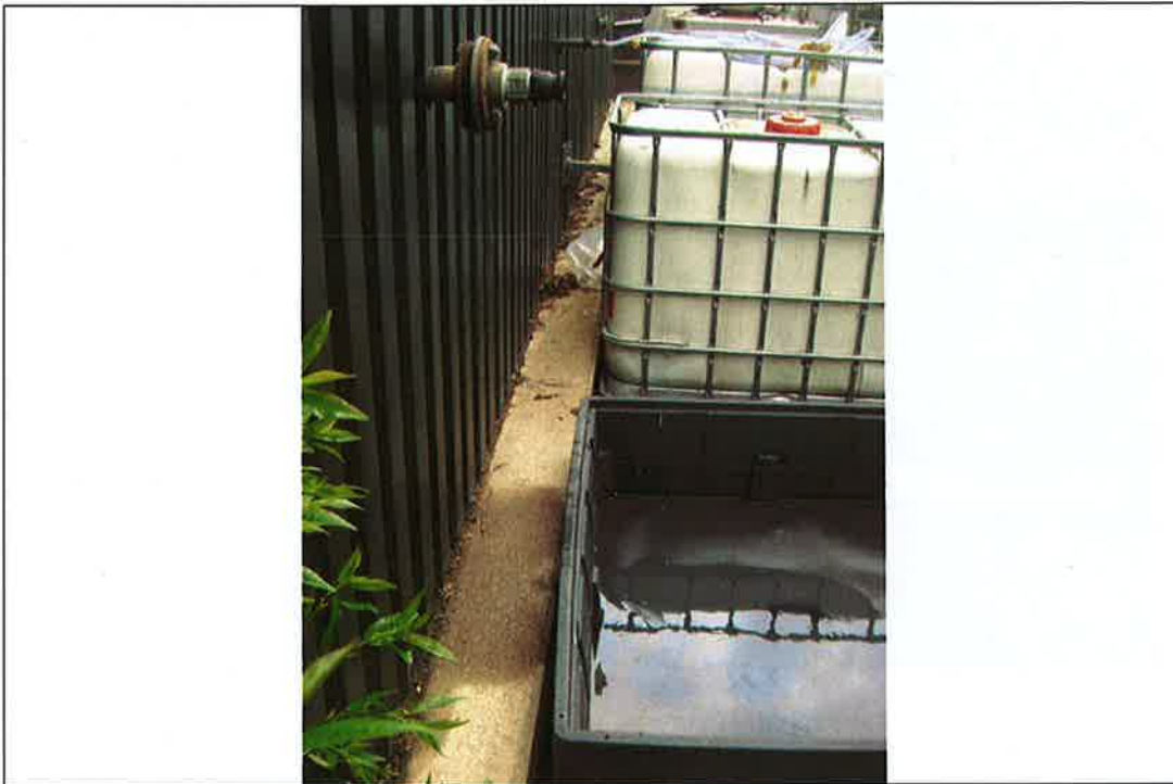
Fig. 27.2: Bund 27 – connection point for acid delivery does not extend over grey Chemstore container
