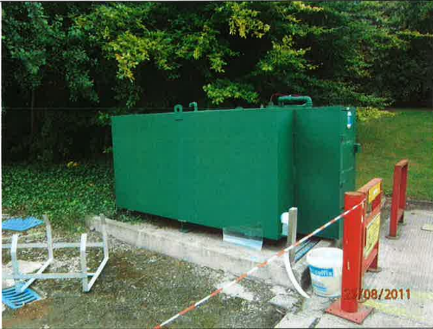
Fig 31.1: Bund 31 - Double-skinned diesel tank refuelling shunters
