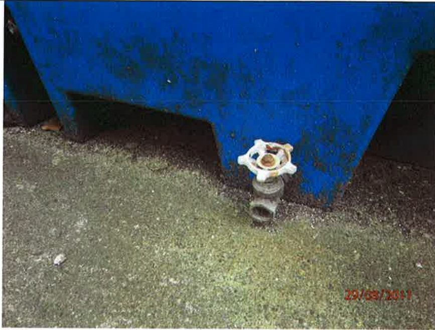
Figure 18.2: Bottom Outlet Valve of Bund 18
