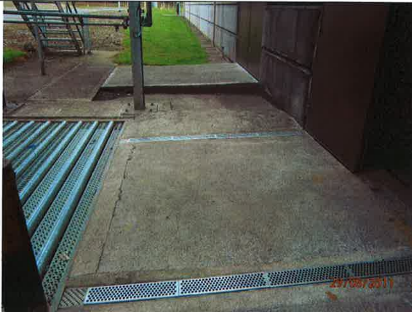
Fig. 23.3: Bund 23 – uncontained area between bund and delivery connection point
