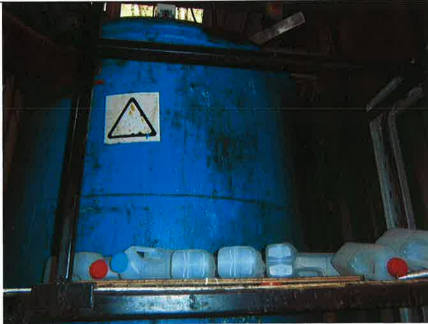
Fig. 24.1: Bund 24 – Mixing tank in bunded area (Tank empty and due for removal)
