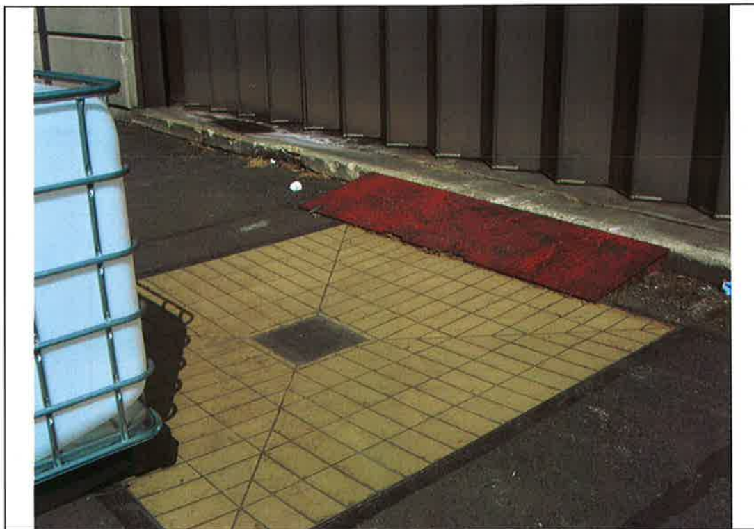
Fig. 32.3: Bund 32 – Effluent drain outside process area on south side
