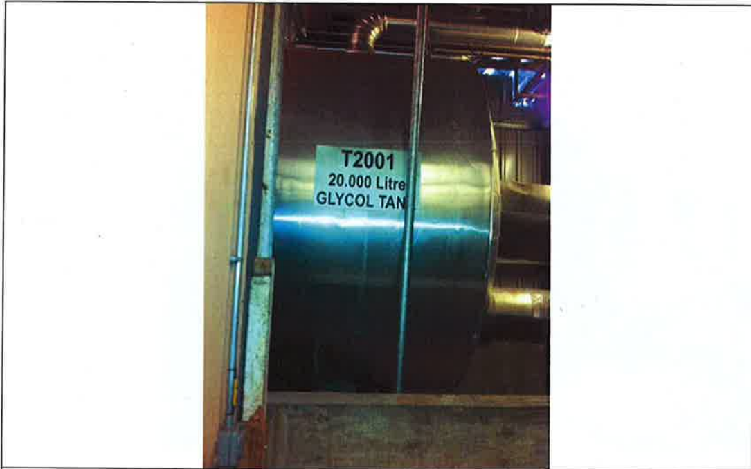
Fig. 41.1: Tank within Bund 41
