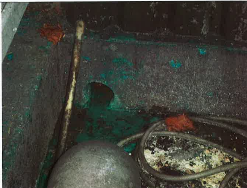
Fig. 24.2: Bund 24 – Hole in SW corner of bund
