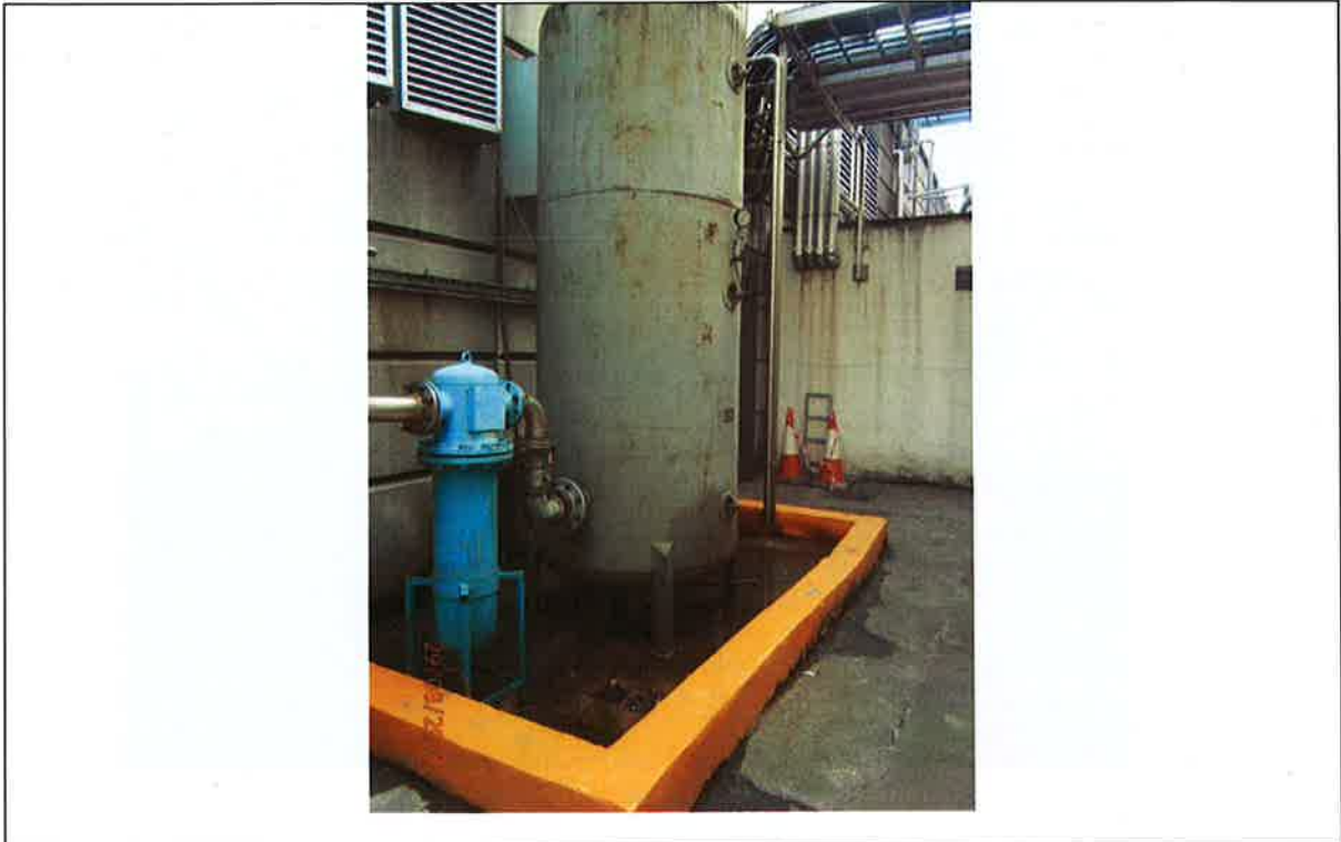
Fig. 20.1: Bund 20 (Note dampness on outside of bund wall)
