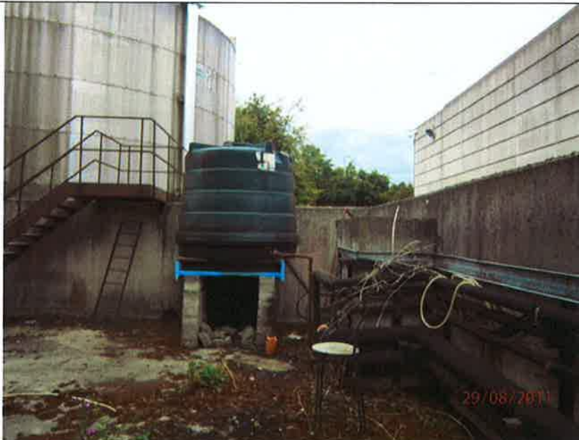
Fig 28.5: Bund 28 – Poor condition of piping associated with the disused diesel bunds; Diesel tank use for periodic testing of boilers
