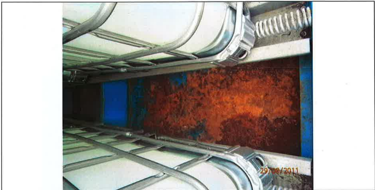
Fig. 14.2: Rusting at base of Bund 14
