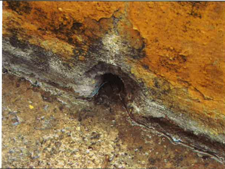
Fig. 8.2: Bund 08 - Hole on NE corner of bund
