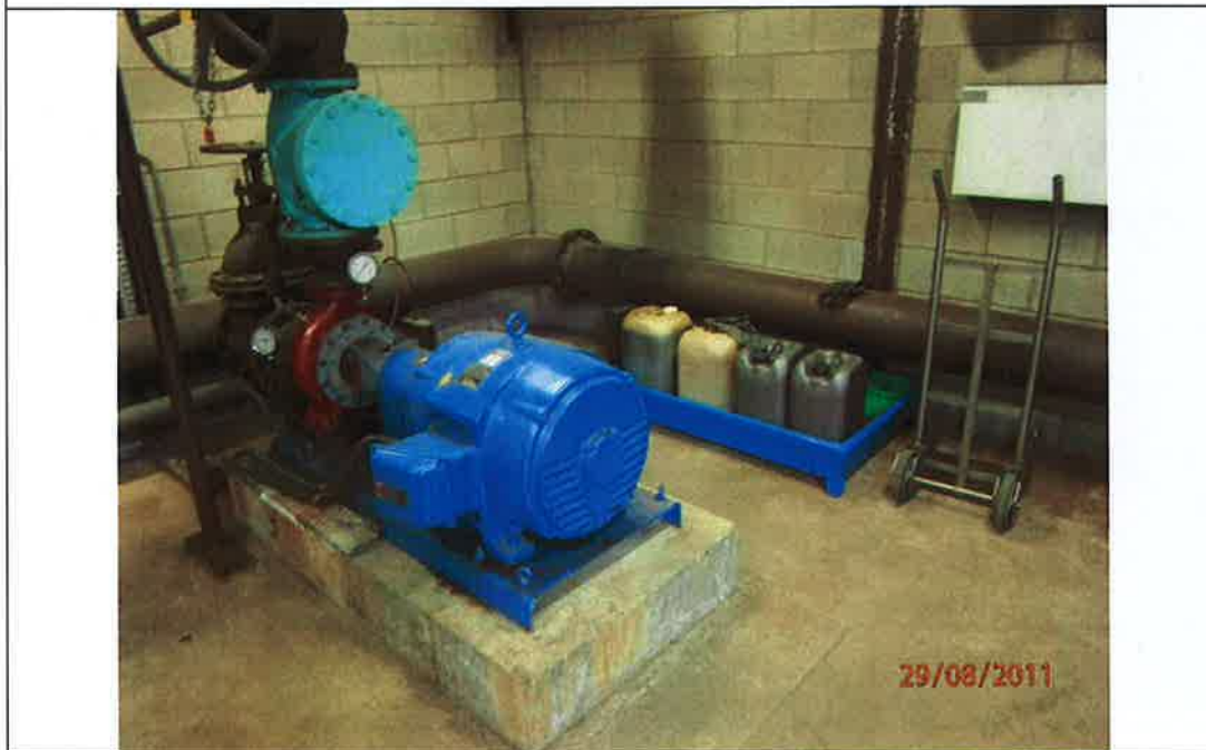
Fig 30.3: Bund 30 – Electric pump at south end of Sprinkler Pump House
