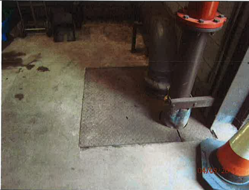
Fig 30.4: Bund 30 – Cover on underground ductway for fire water pipes
