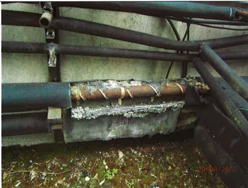
Fig 28.3: Bund 28 – Poor condition of pipework within bund
