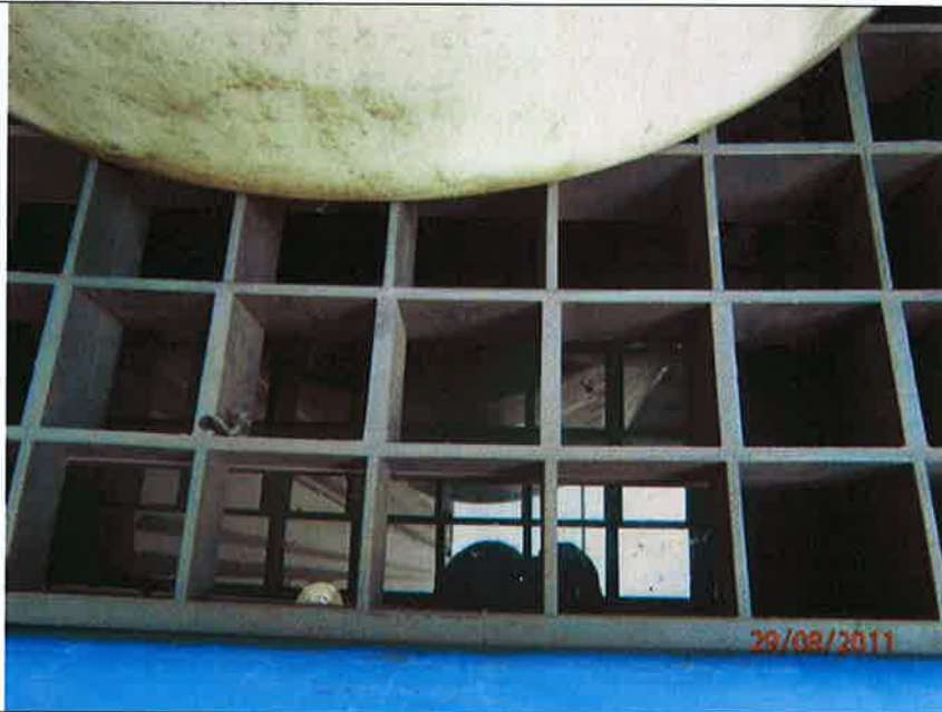
Fig. 18.3: Liquid within Bund 18 reducing bund capacity (same applies to Bund 19)
