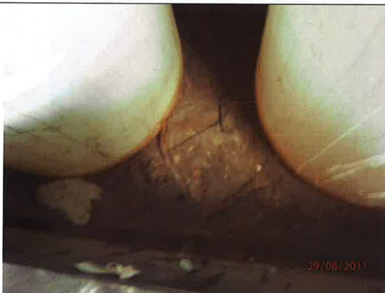
Fig 29.2: Bund 29 - Debris in base of bund
