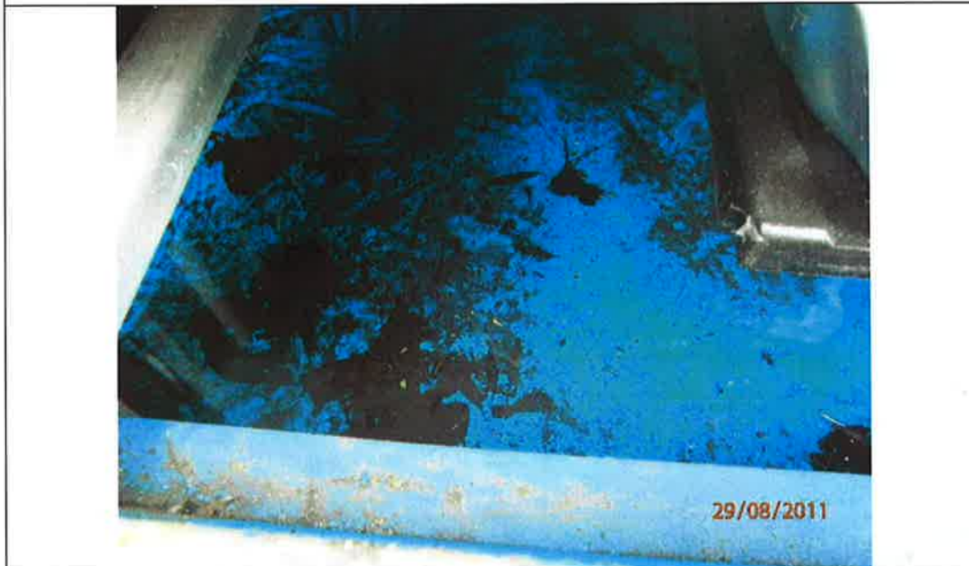
Fig. 33.2: Liquid present in base of bund
