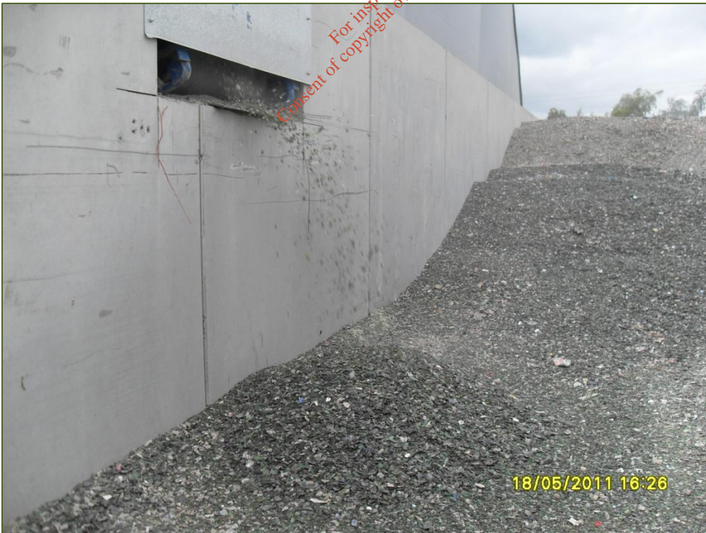
Photograph D.2.10: Output from the Drying Plant for diversion to Main Process
