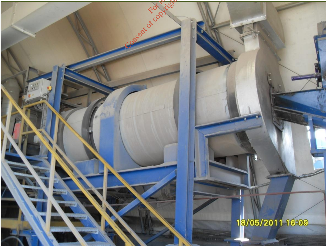
Photograph D.1.6: Rotating Drying Unit
