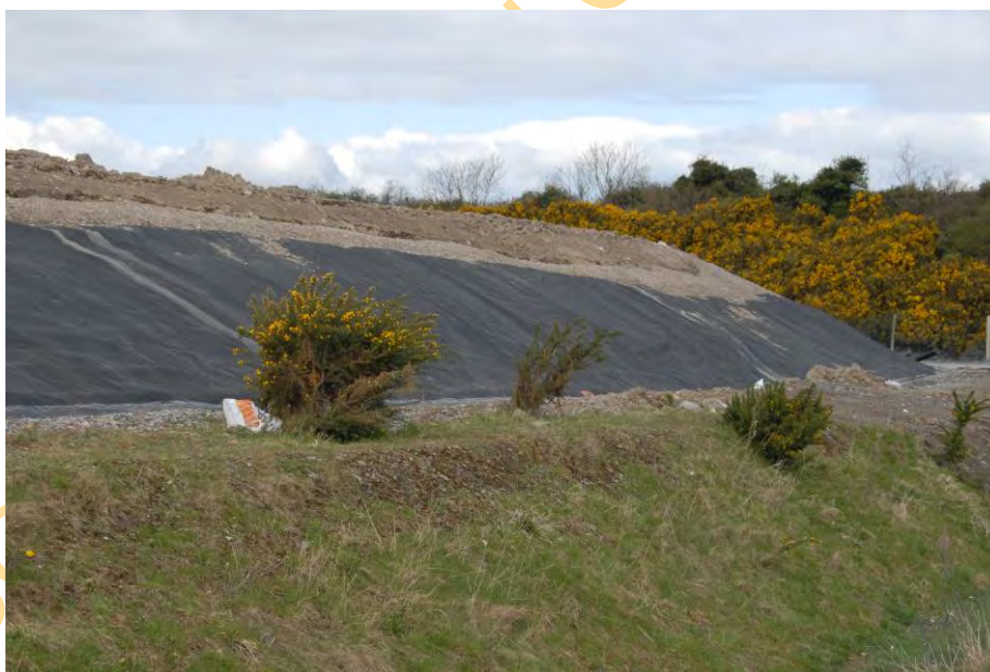
Plate 2: Partial capping material placed on side slopes at the rear of Cell 15. HDPE Liner welded to anchor trench.
