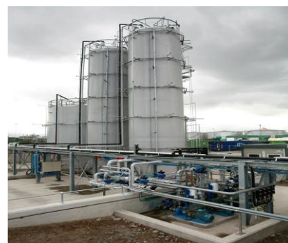
Figure 1.2.3 Picture of Tank Farm
