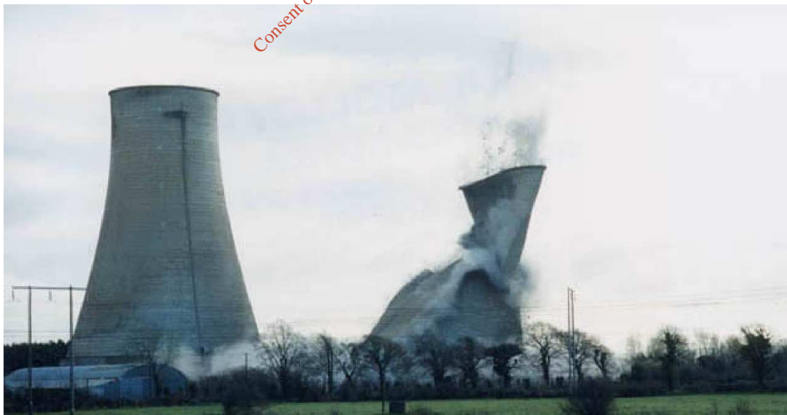
Figure 2.6 Demolition of the First Cooling Tower at the Former Ferbane Peat Fired Station
