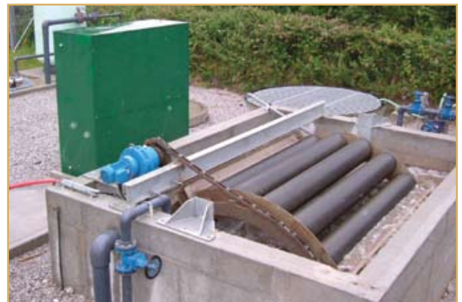
WWTW Shanagary, Ireland for 600 P.E
