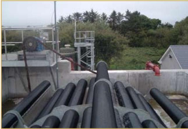
WWTW Carney, Ireland for 2500 P.E.
