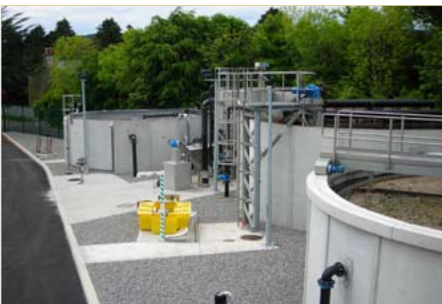
WWTW Coolaney, Ireland for 2500 P.E.
