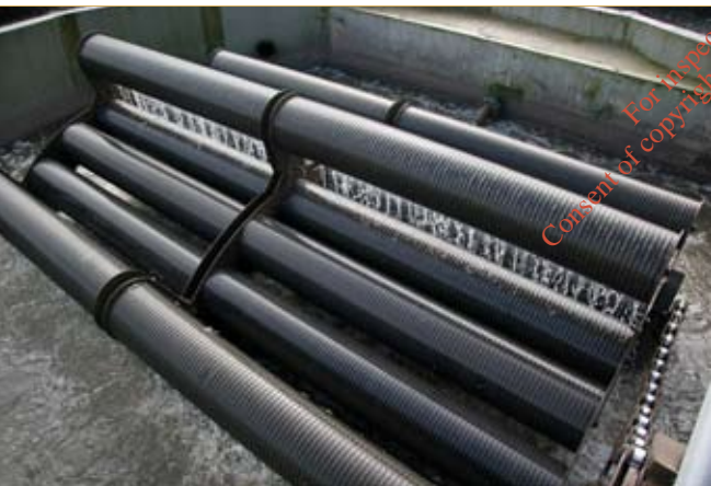
WWTW Doonbeg, Ireland for 1500 P.E.
