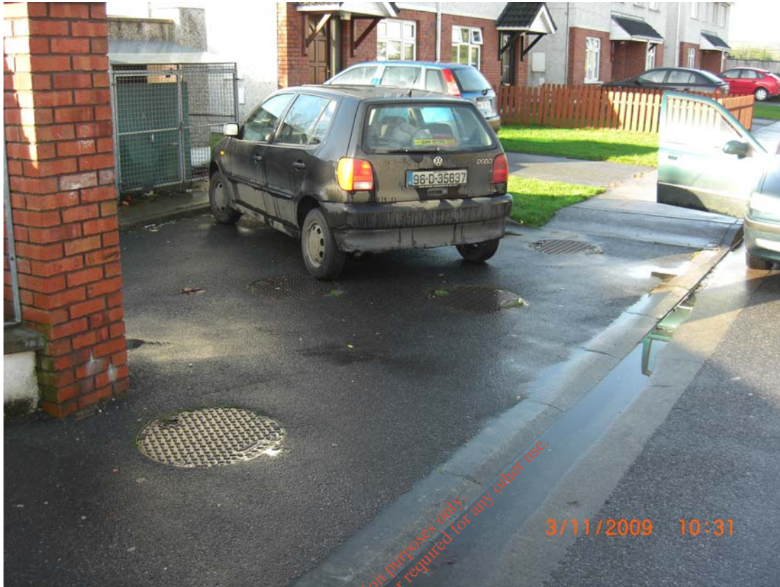
Photo – KK-WWDL-213-C.1.2.1 – Pumping Station Nuenna Court
