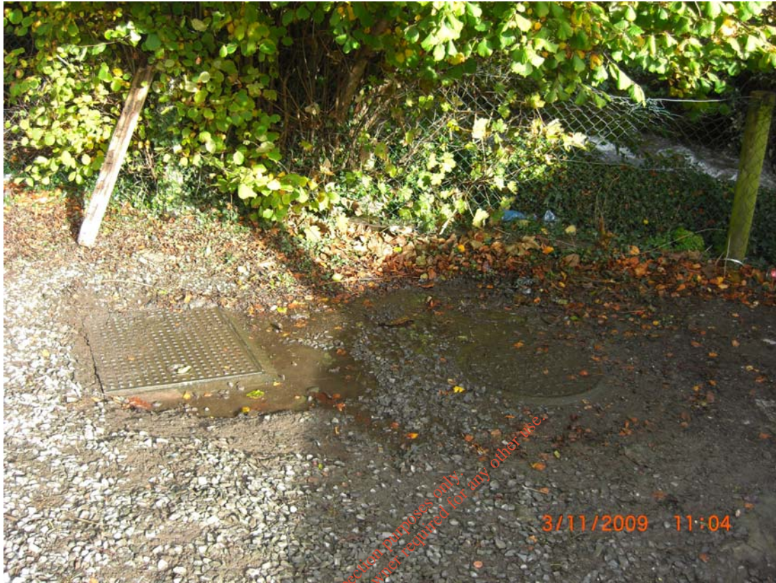
Photo – KK-WWDL-213-C.1.2.1 – Pumping Station Nuenna Court
