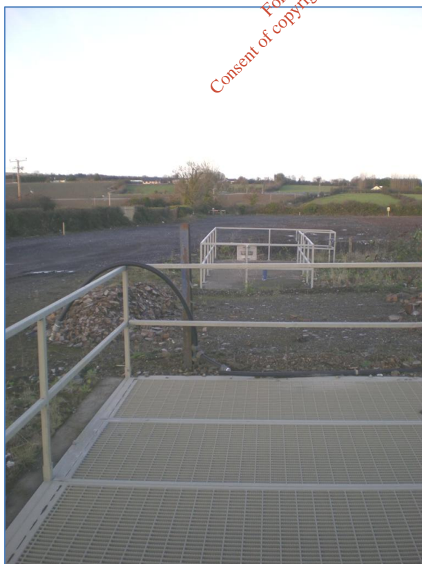
Photograph D.13: Surface Water Management Inspection Chamber (existing infrastructure)
