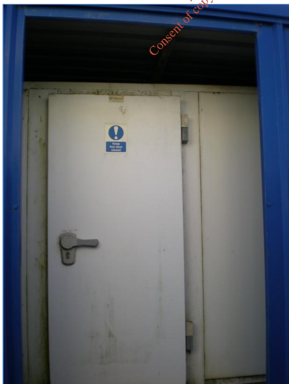
Photograph D.9: Refrigerated Sample Storage Unit (existing infrastructure)
