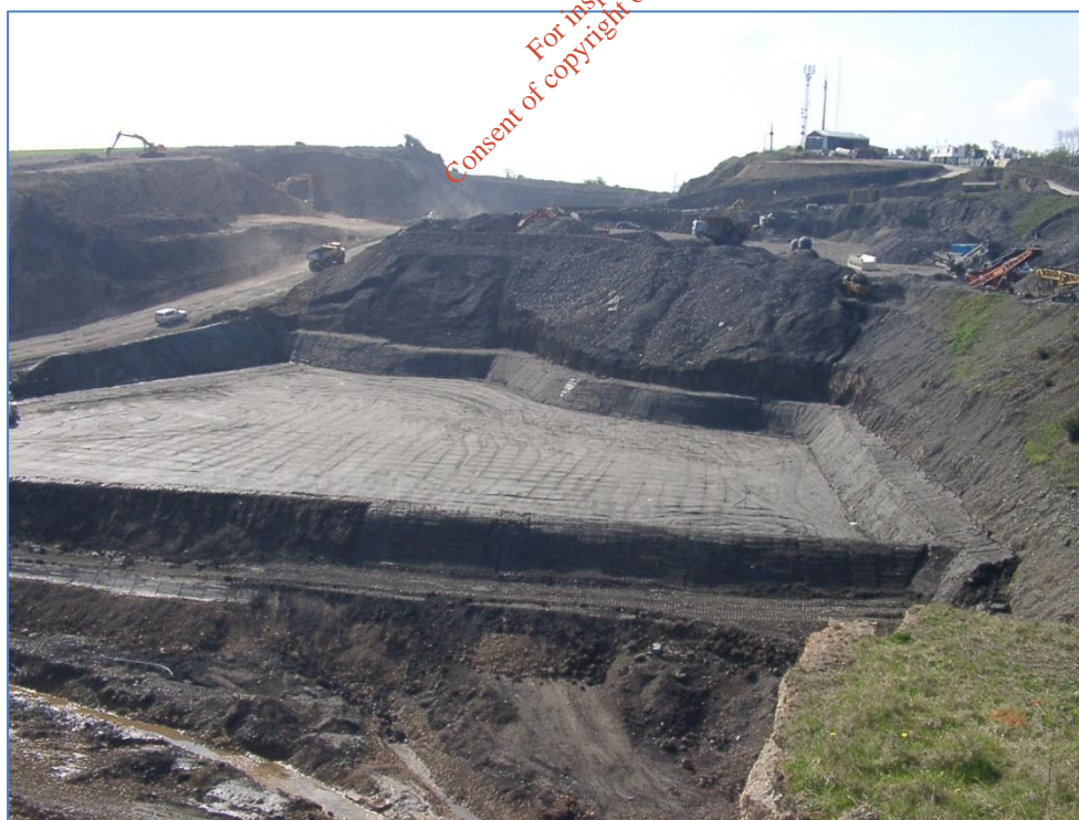
Photograph D.17: First MEHL inert cell, prior to waste deposition (existing infrastructure)
