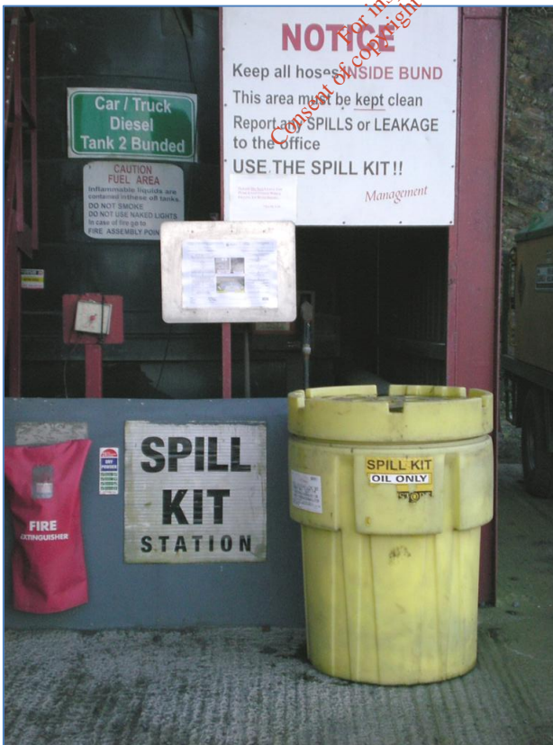
Photograph D.11: Spill Control Equipment (existing infrastructure)
