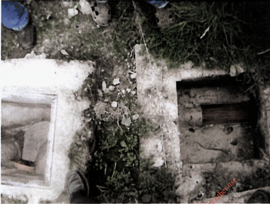
Photograph 1: Storm water monitoring point SW1, and adjacent manhole, at south eastern side of unit
