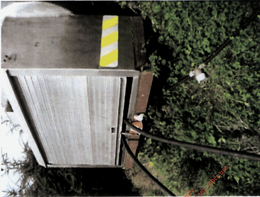
Photograph 5: Water Meter for well AGW2
