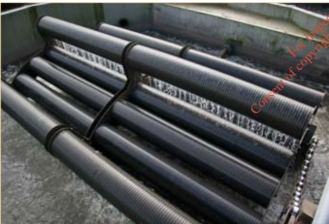
WWTW Doonbeg, Ireland for 1500 P.E.
