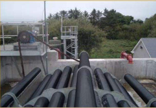
WWTW Carney, Ireland for 2500 P.E.
