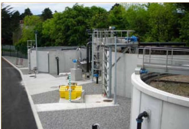
WWTW Coolaney, Ireland for 2500 P.E.
