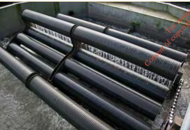
WWTW Doonbeg, Ireland for 1500 P.E.
