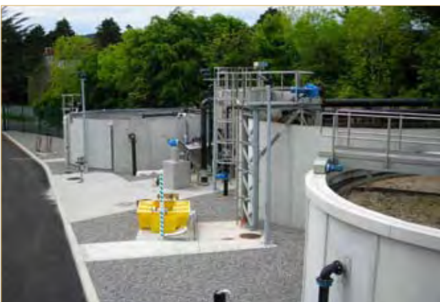
WWTW Coolaney, Ireland for 2500 P.E.
