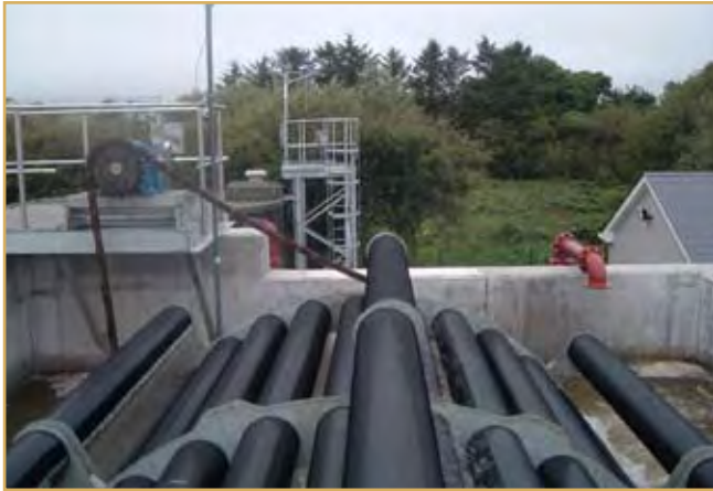
WWTW Carney, Ireland for 2500 P.E.
