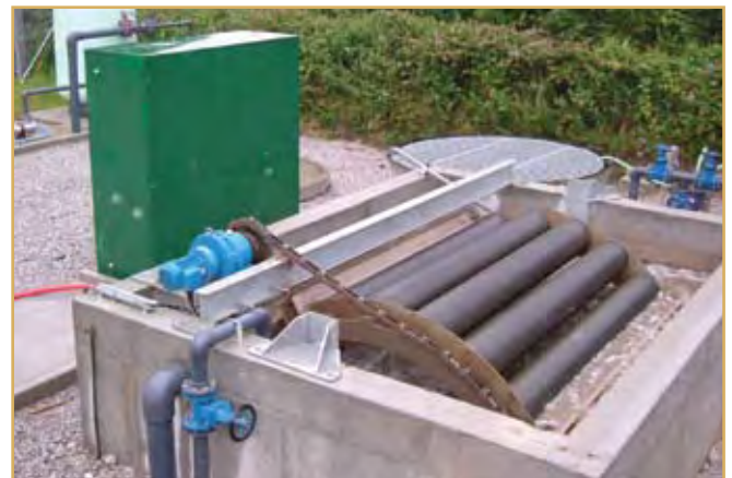
WWTW Shanagary, Ireland for 600 P.E
