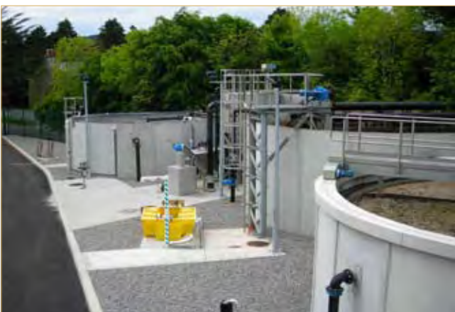
WWTW Coolaney, Ireland for 2500 P.E.
