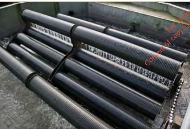
WWTW Doonbeg, Ireland for 1500 P.E.
