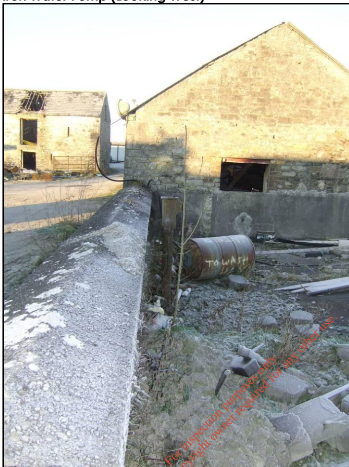
Plate 16.33: BH6, Northern Elevation Wall abutting Outbuilding 1 showing Cast Iron Water Pump (Looking West)
