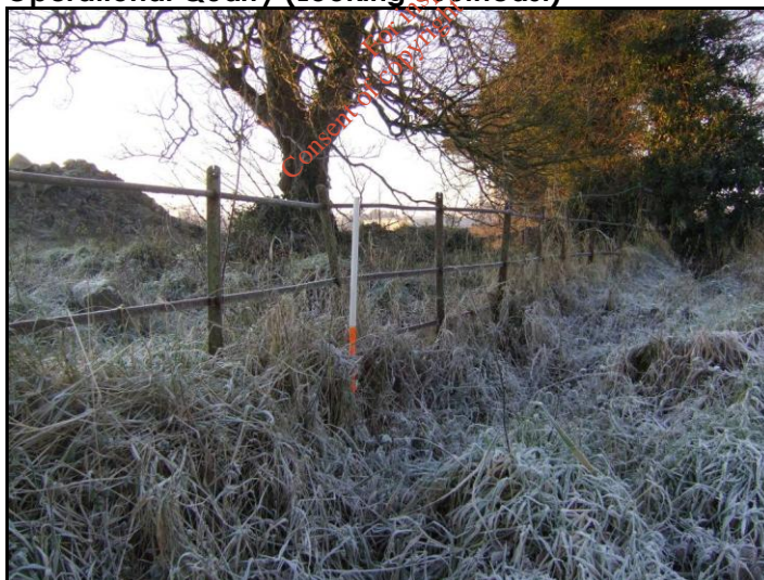
Plate 16.44: BH7, Original Iron Avenue Railings along Western Extent of Operational Quarry (Looking Southeast)
