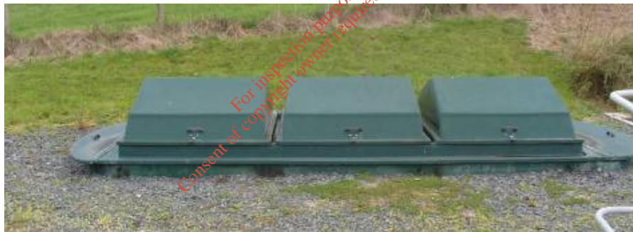
Photograph 3 Rotating Biological Contactor
