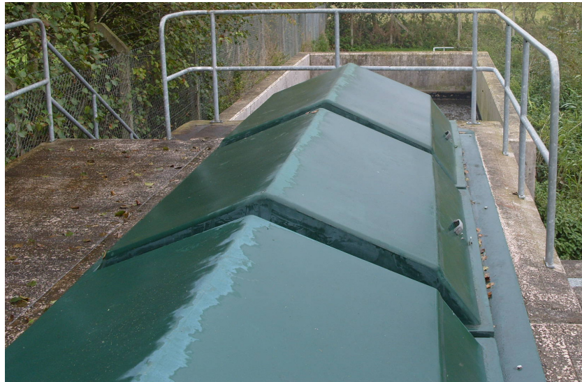
Photograph 2 Rotating Biological Contactor
