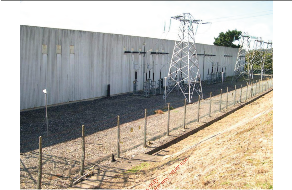
Location No: 23 View southwest 110 kV switching yard.
