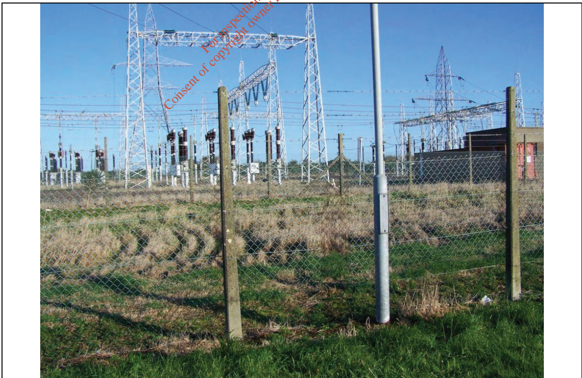
Location No: 22 View north 220kV switching yard.
