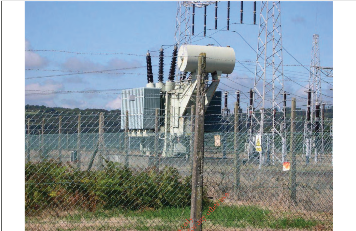
Location No: 22 View northwest 220kV switching yard.
