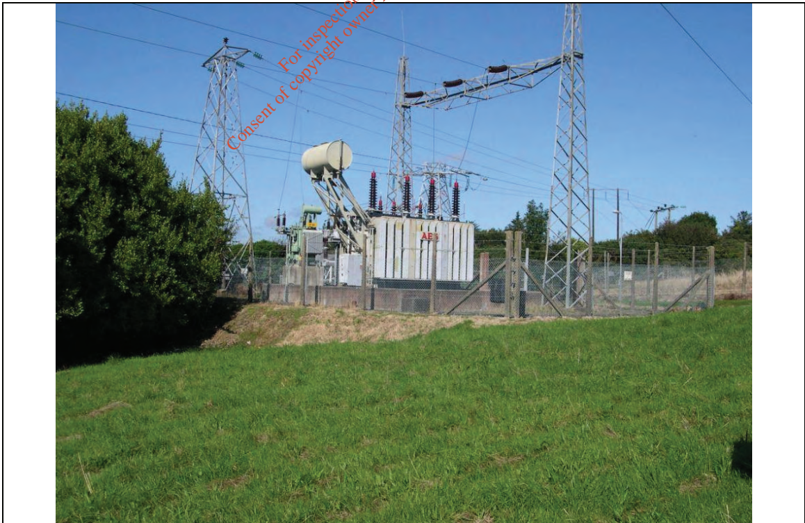
Location No: 24 View northwest 110 kV switching yard.
