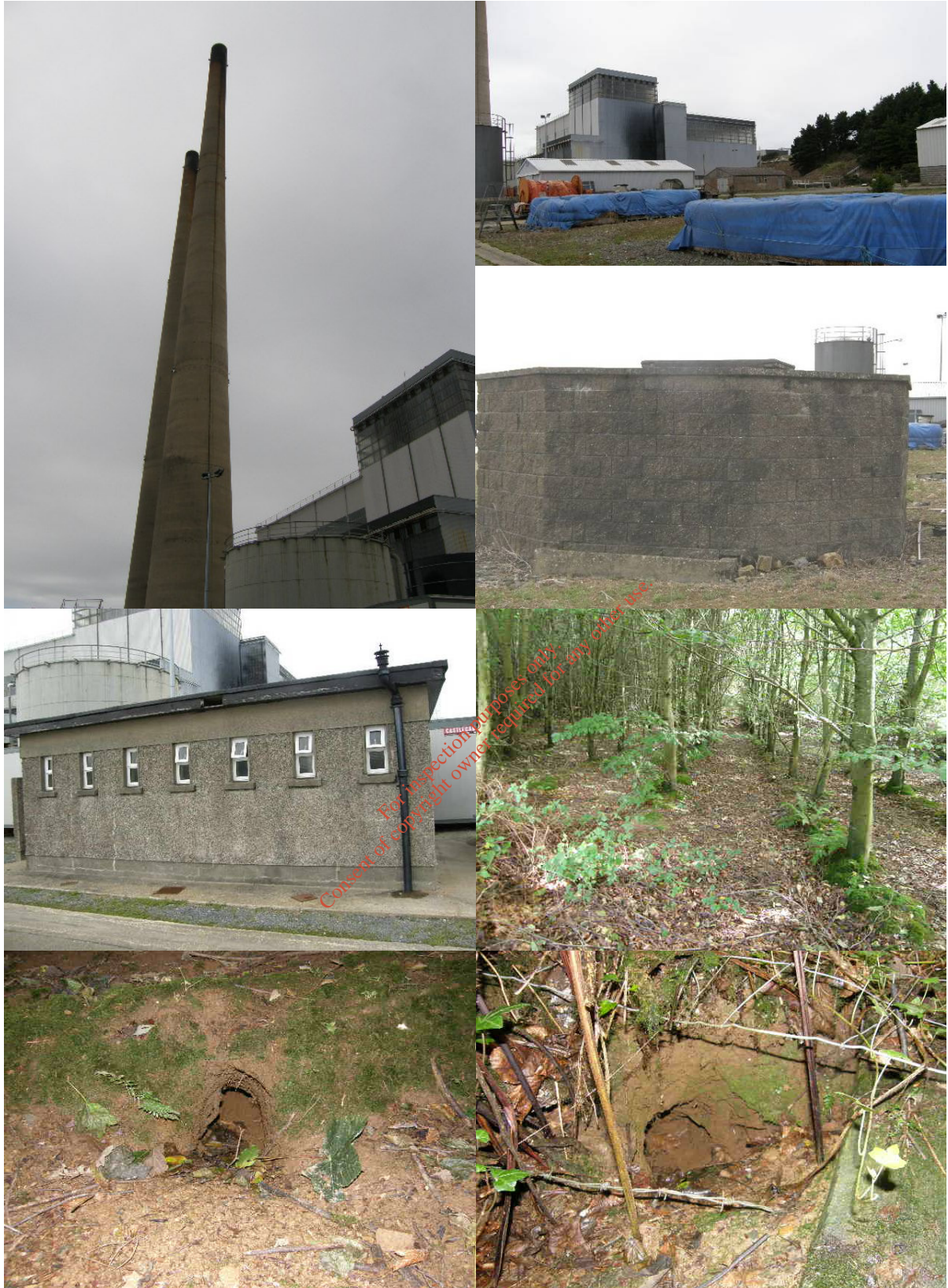
Plate 4: Buildings with roost potential but no bats and sites in the woods with rabbit warrens
