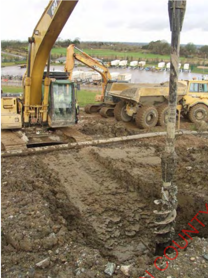
Plate:3 : Auger attached to CAT Excavator. Drilling of new gas wells as deemed necessary by Facility Manager.
