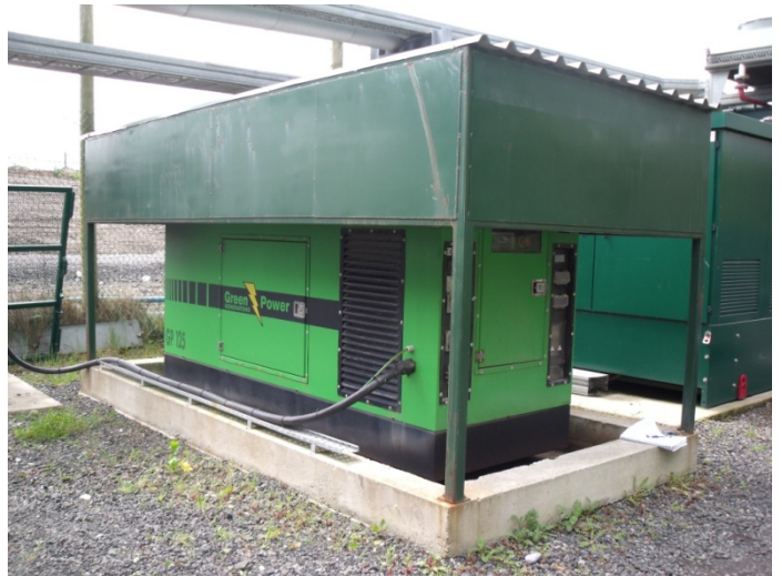
Photo 4: Concrete Bunded Tank (GP125 Generator)
