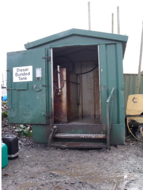
Photo 3: Walk in Diesel Tank
