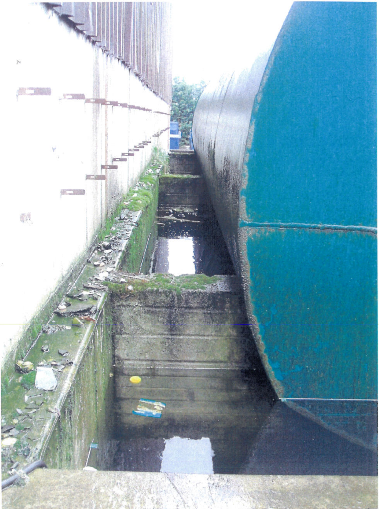
Photo No.2 View of diesel oil tank bund full of water.
