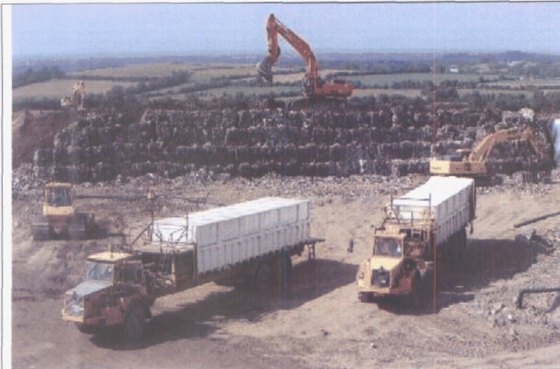
Photograph showing Arthurstown baled-waste landfill, waste placement machine at bottom of face, cover machine on top
