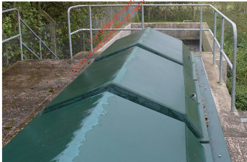
Photograph 2 Rotating Biological Contactor
