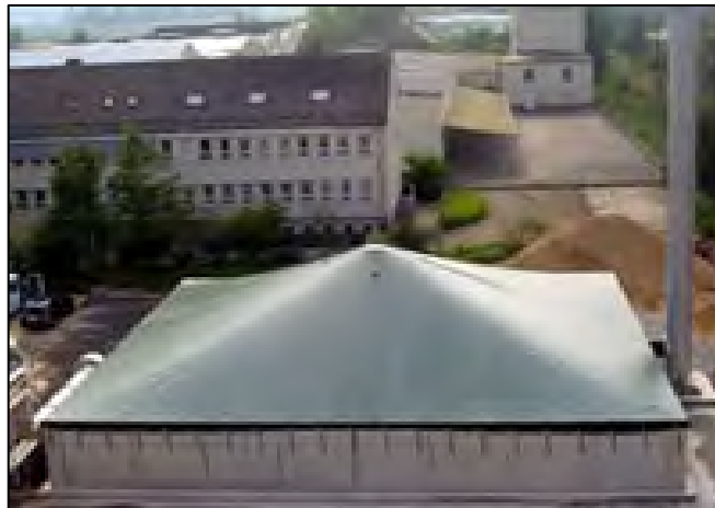
Figure 1: Typical enclosed Biofilter with Stack
