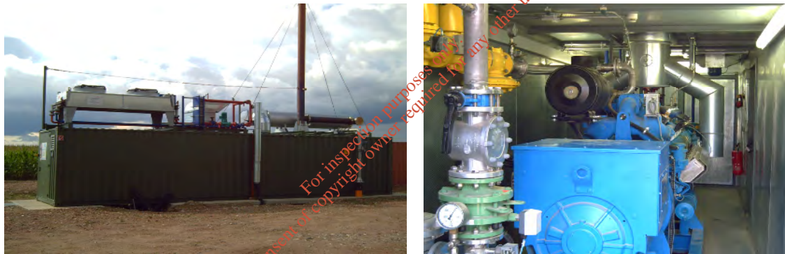
Fig. 13. Containerised CHP at the Decker biogas plant in Northern Germany
