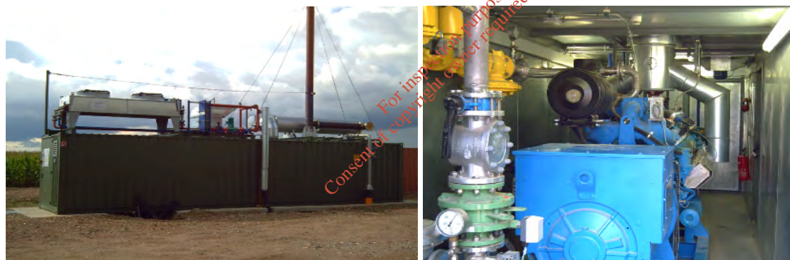
Fig. 14. Containerised CHP at the Decker biogas plant in Northern Germany
