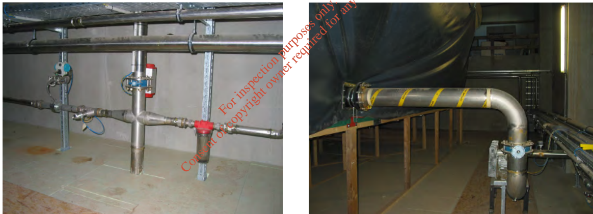
Fig. 12. The pneumatic gas collection system on the roof of the fermenters (left) and the gas transfer blower to the gas bag located in the roof space above the fermenters (right).
