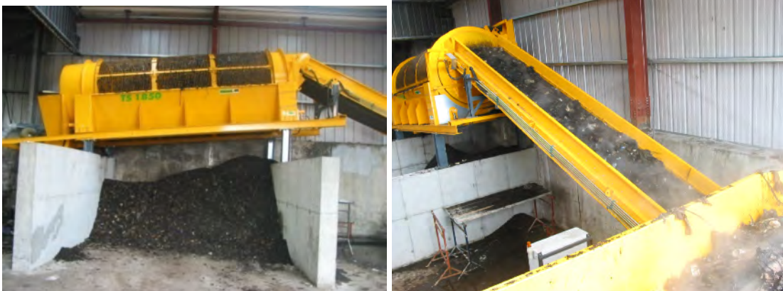
Fig. 18. Housed trommel screen illustrating multiple sections that produce different grades of compost and overs.
