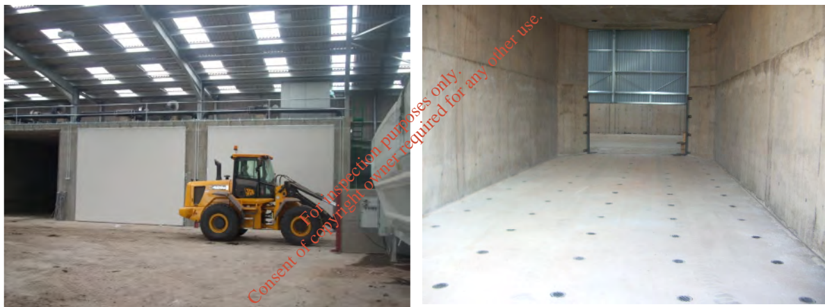
Fig. 14. Exterior of the composting biocells illustrating the sliding doors (left) and the proprietary C:N in-pavement aeration system (right).
