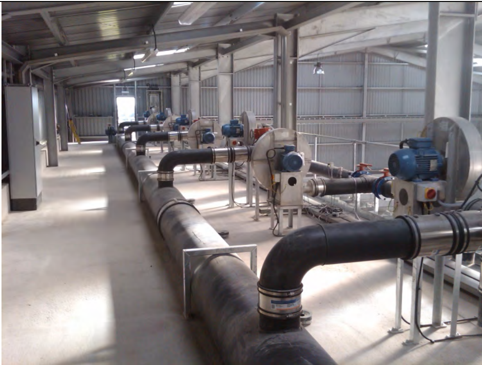
Fig. 17. The blower modules in the gallery of the Deepmoor tunnel composting facility in Devon.
