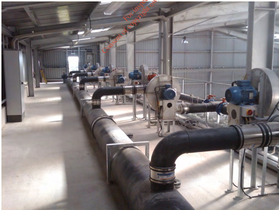
Fig. 16. The blower modules in the gallery of the Deepmoor tunnel composting facility in Devon.
