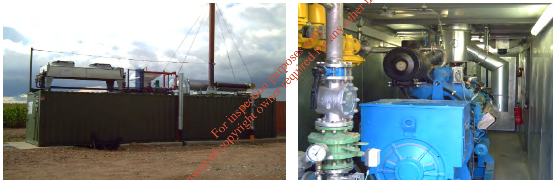
Fig. 13. Containerised CHP at the Decker biogas plant in Northern Germany
