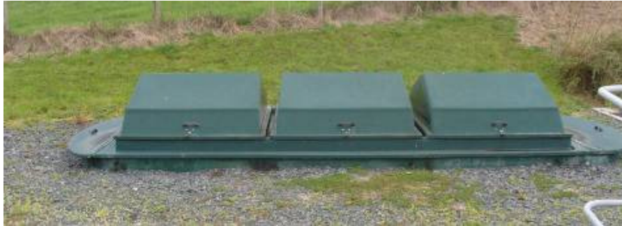
Photograph 3 Rotating Biological Contactor
